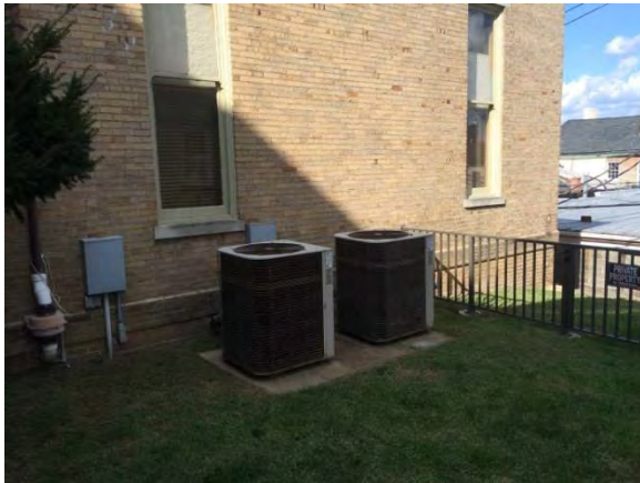
Figure 5.10: Library condensing units.
