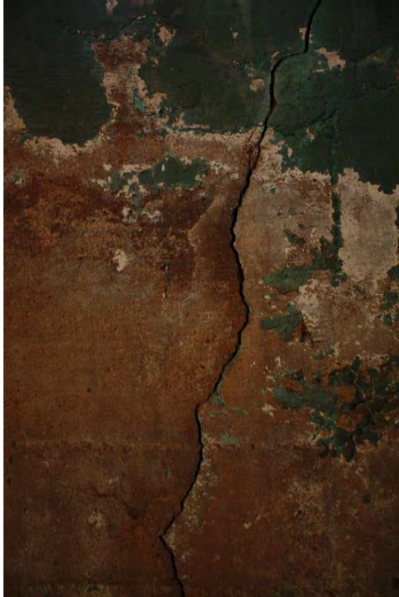
Figure 3.380, Old Jail, Basement, Room 005, detail view of a vertical crack underneath the window at the north wall.
