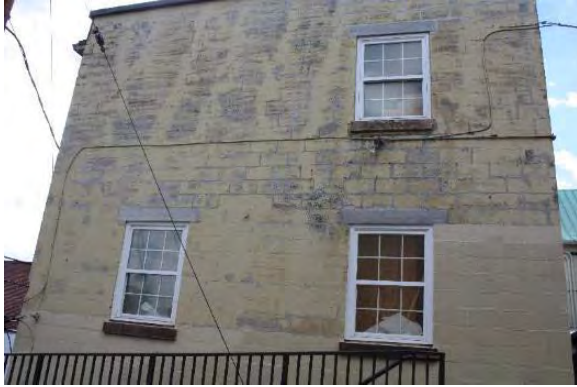
Figure 3.332, Old Jail, north elevation, general view looking south. Note the large areas of paint loss at the wall.
