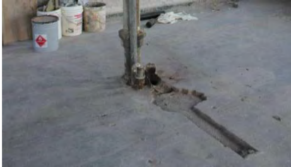
Figure 3.449, Old Jail, Second Floor, Room 201, view of marks from a former sanitary line at the north end of the room.
