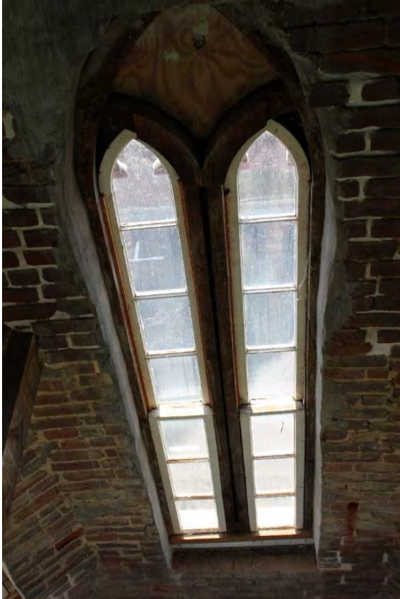
Figure 3.203, Historic Courthouse, Bell Tower, Room 302, view of a third-story window. Note the Portland Cement based mortar patching.
