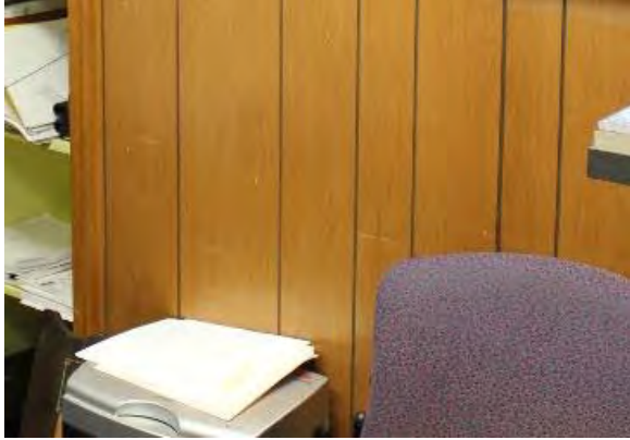
Figure 3.284, Old Wallace Library, First Floor, Room 107, detail view of minor scratches at faux wood paneling.
