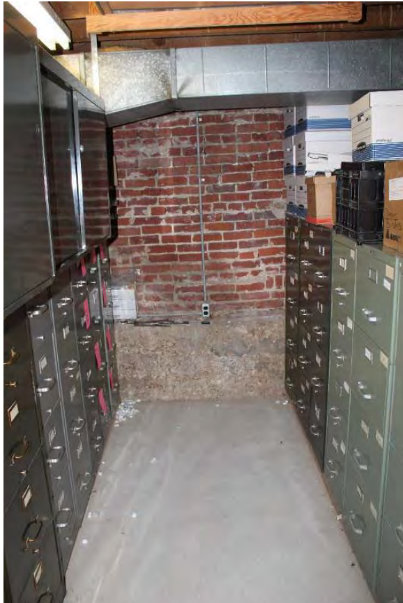
Figure 3.245, Old Wallace Library, Basement, Room 001, general view looking north. Note the transition of wall material from concrete at the base to brick above.
