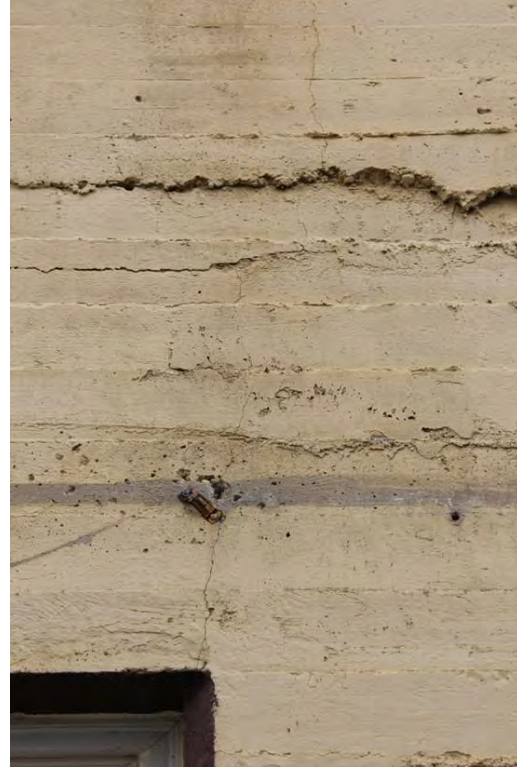
Figure 1.16, Old Jail. Cracking of the exterior concrete wall surfaces. Photograph 2015.
