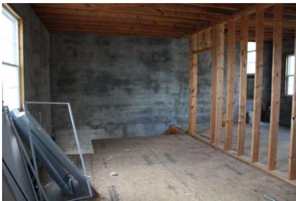
Figure 3.454, Old Jail, Second Floor, Room 202, general view looking south in the east end of the room. Note that the floor is open to the stairwell below and there is no railing, posing a safety hazard. Also note the unfinished wall framing dividing the room.
