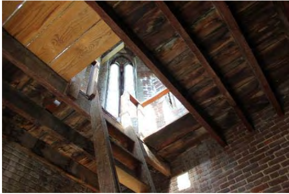
Figure 3.201, Historic Courthouse, Bell Tower, Room 302, view of the ceiling at the second story, looking up through the access hatch to the third story.
