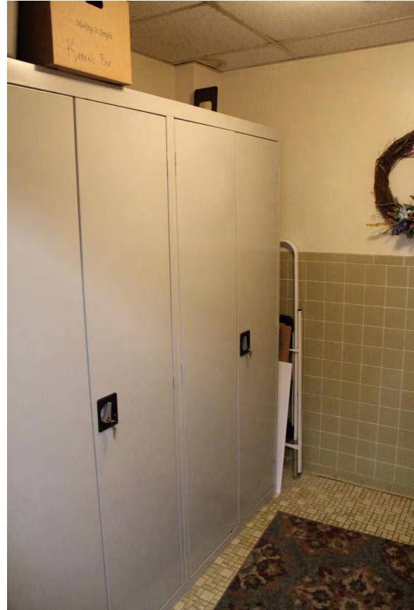
Figure 3.310, Old Wallace Library, Second Floor, Room 207, view looking southeast toward lockers. The lockers obscure a window at the east wall.
