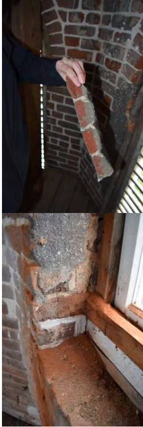
Figure 4.44: Deteriorated brick in and delaminating parging at Bell Tower window jambs
