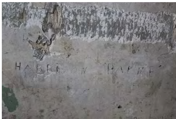
Figure 3.411, Old Jail, First Floor, Room 106, view of graffiti at the wall.
