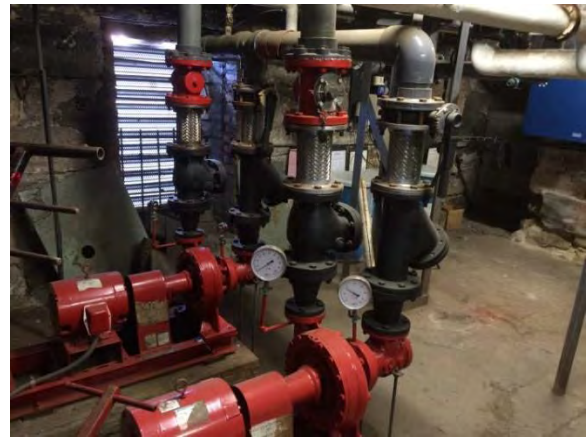
Figure 5.2: Pumps in Old Jail Basement
