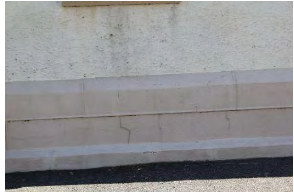
Figure 3.25, Historic Renwick Courthouse, east elevation, detail view of foundation. Note the extruded mortar joints and the vertical crack.
