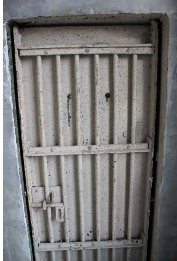
Figure 3.402, Old Jail, First Floor, Room 104, view of the jail cell door at the north wall of the east vestibule. Note the paint crazing and rusting throughout.
