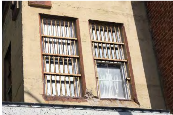
Figure 3.353, Old Jail, south elevation, view of second-story windows west of the chimney. Note the missing sills at both windows and removed bars at the east window. The concrete is spalling where the sills were formerly located.
