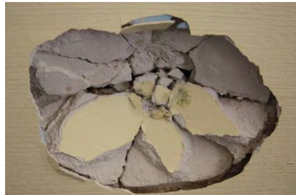
Figure 3.68, Historic Courthouse, First Floor, Room 115, view of hole in east plaster wall.
