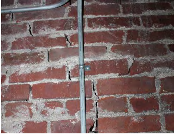
Figure 3.248, Old Wallace Library, Basement, Room 001, view of a step crack at the north wall.
