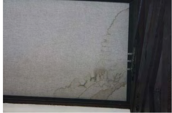
Figure 3.150, Historic Courthouse, Second Floor, Room 212, view of moisture staining at the acoustic paneling.
