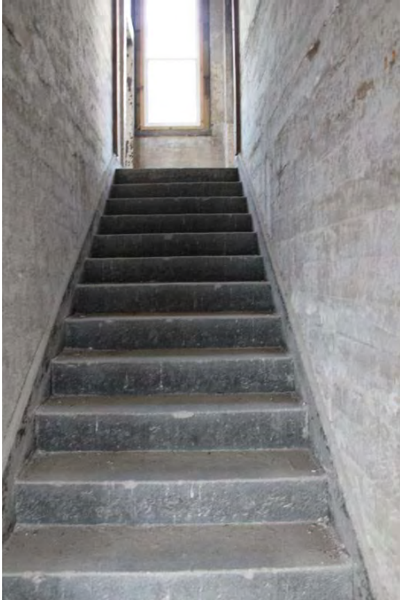
Figure 3.422, Old Jail, First Floor, Room 108, view of stair from first story; note the small areas of loss at the ends of the treads.
