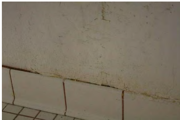
Figure 3.131, Historic Courthouse, Second Floor, Room 204, view of damage to south wall under urinal.
