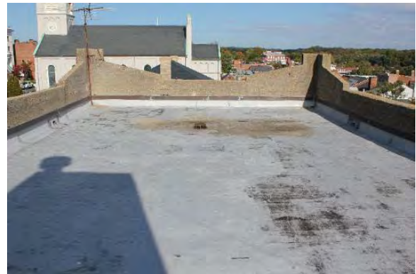
Figure 3.320, Old Jail, roof, view of higher flat membrane roof looking south. Note the parapets.
