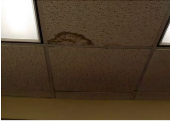
Figure 3.63, Historic Courthouse, First Floor, Room 112, view of moisture staining at the ceiling toward the center of the room.
