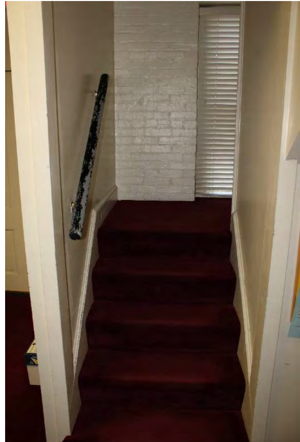
Figure 3.289, Old Wallace Library, First Floor, Room 109, view of lower flight of stairs. Note the heavy paint loss at the handrail.
