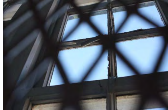
Figure 3.185, Historic Courthouse, Second Floor, Room 221, view of paint failure at the muntins of the north window.
