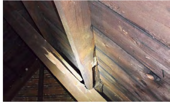
Figure 4.15: Splintered purlin and truss top chord, rumored to be due to cannon ball damage
