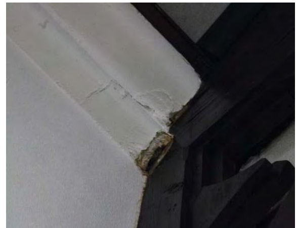
Figure 3.152, Historic Courthouse, Second Floor, Room 212, view of cracks at the crown molding in the southeast corner of the room.
