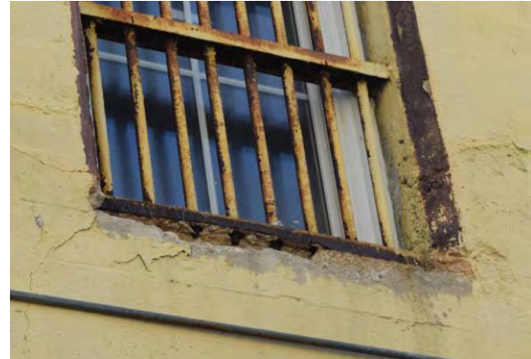
Figure 4.64: Spalled concrete and missing sill at second floor window opening on west façade
