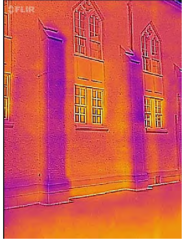
Figure 3.27A, Historic Renwick Courthouse, east elevation, infrared view of butresses. Note how much cooler in color the butresses are. This could be due to moisture sitting on the projecting surfaces.
