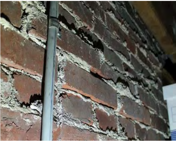
Figure 3.249, Old Wallace Library, Basement, Room 001, view of uneven mortar at the north wall.
