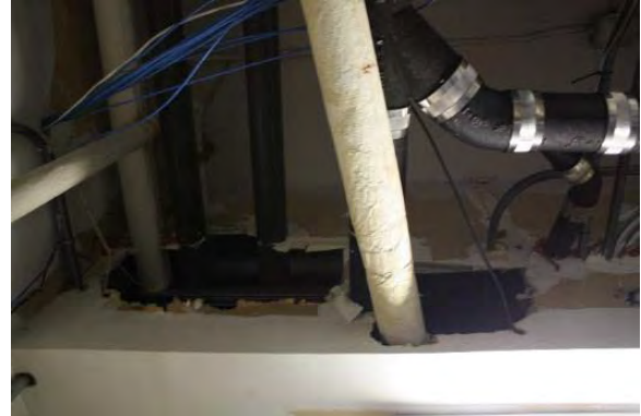
Figure 3.60, Historic Courthouse, First Floor, Room 108, view of holes cut in drywall for pipes.
