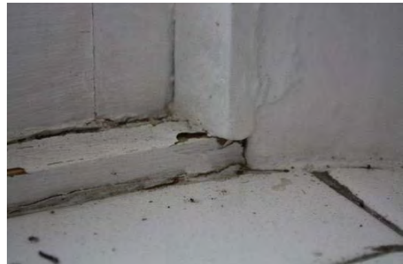
Figure 3.175, Historic Courthouse, Second Floor, Room 217, view of paint loss and damage at the wood window frame.
