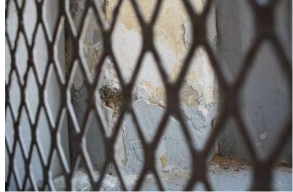
Figure 3.190, Historic Courthouse, Second Floor, Room 222, view of efflorescence and paint failure at a window reveal.
