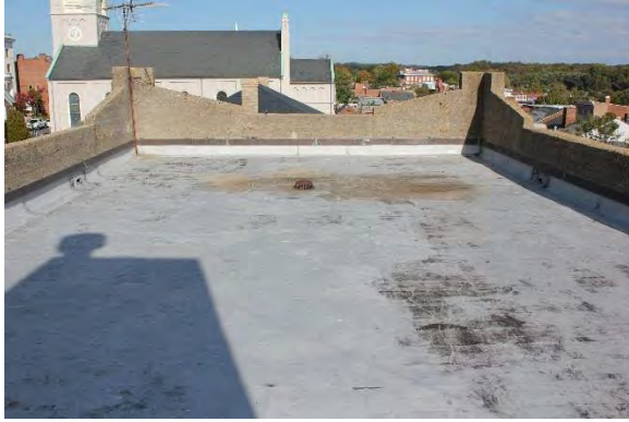
Figure 1.18, Old Jail roof, which is nearing the end of its expected lifespan. Photograph 2015.
