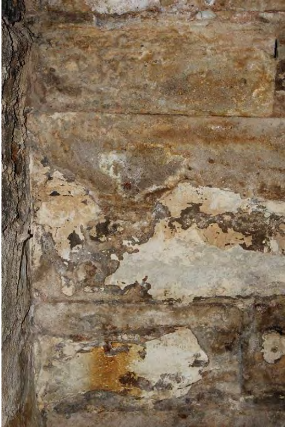
Figure 3.361, Old Jail, Basement, Room 002, detail view of efflorescence and moisture staining at stone walls.
