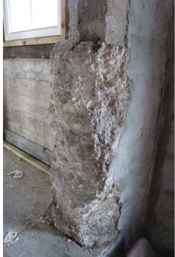
Figure 3.448, Old Jail, Second Floor, Room 201, detail view of the rough-cut opening between Rooms 201 and 202.
