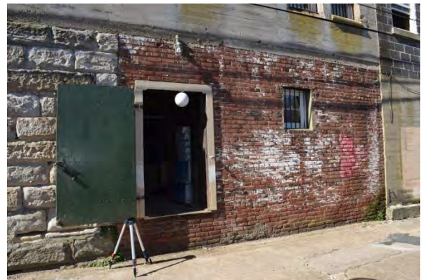
Figure 4.62: Historic brick and ashlar stone masonry foundation walls at southern and central portions and cast-in-place foundation wall at northern portion of jail
