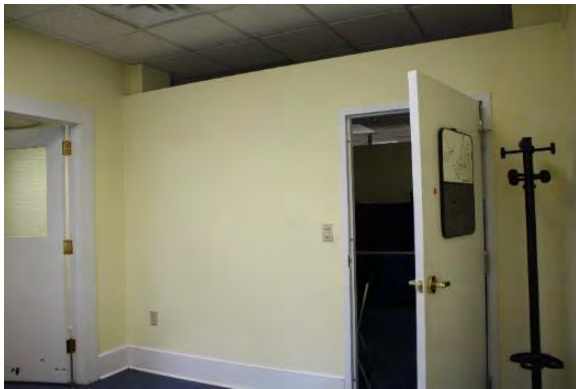
Figure 3.84, Historic Courthouse, First Floor, Room 120, general view looking east. Note that the partition wall that does not meet the ceiling.
