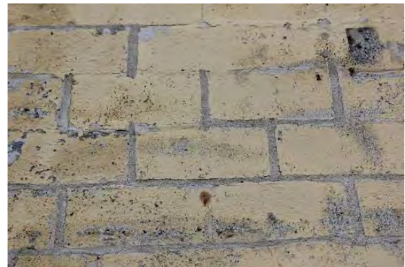
Figure 3.323, Old Jail, west elevation, detail view of painted concrete block wall. Note the areas of paint loss.
