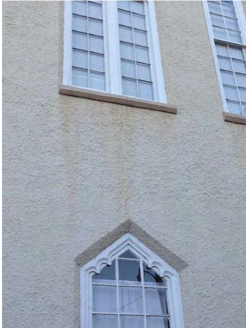
Figure 4.07: East façade with stucco cracking between windows.
