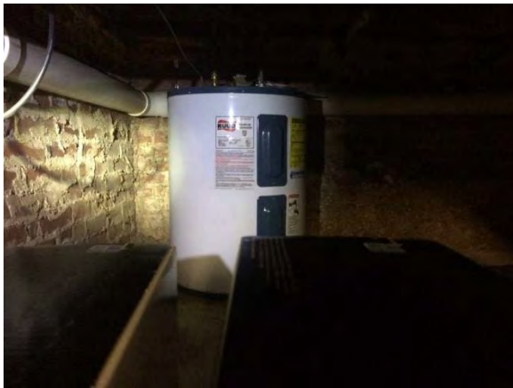
Figure 5.16: Library, electric water heater.
