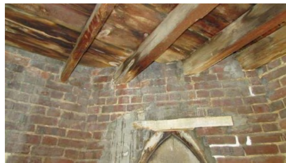
Figure 19: Bell floor joist bearing deterioration
