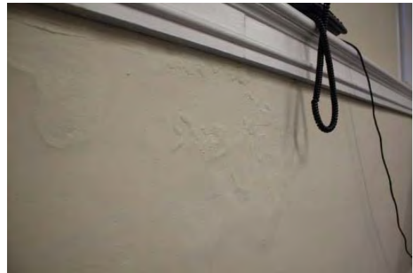
Figure 3.93, Historic Courthouse, First Floor, Room 123, view of plaster damage underneath the west window of the north wall.
