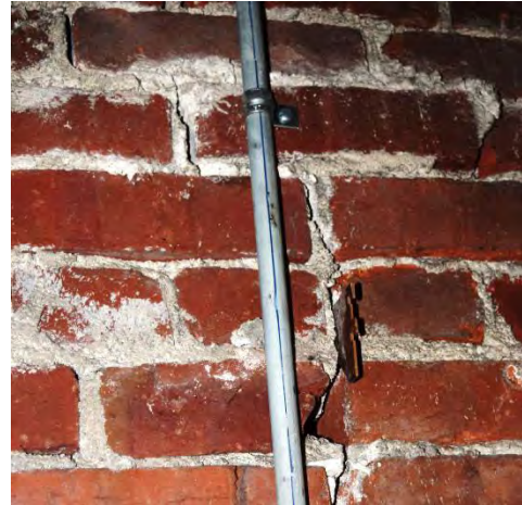
Figure 4.57: Through-wall crack on interior face of north foundation wall. Note shim inserted in crack.
