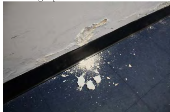
Figure 3.105, Historic Courthouse, First Floor, Room 128, detail view of plaster damage and efflorescence at east wall.
