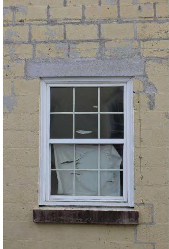
Figure 3.325, Old Jail, west elevation, view of a typical vinyl replacement window at the low-roofed north section.
