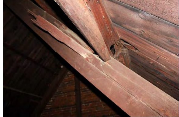
Figure 1.2, Fredericksburg Courthouse, North attic. Shifting of and damage to structural members. Photograph 2015.
