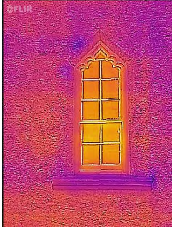
Figure 3.16A, Historic Renwick Courthouse, infrared detail of window. Note the cooler hue on the window sill and upper left near cracking in the stucco. This may be due to water sitting on these surfaces and soaking in through the cracks.
