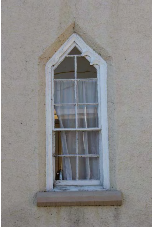
Figure 3.29, Historic Renwick Courthouse, east elevation, view of a typical first-story window; note that this window is missing part of its carved, decorative head, exhibits paint loss, and has a crack at the sill.
