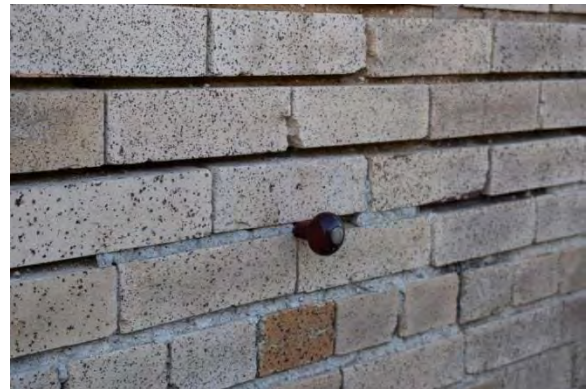
Figure 4.54: Horizontal open mortar joints at east facade of Wallace Library
