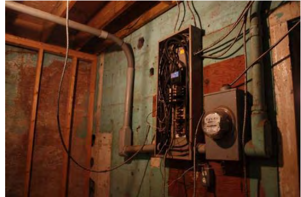
Figure 3.375, Old Jail, Basement, Room 004, view of the electrical panel and exposed wiring at the north wall.
