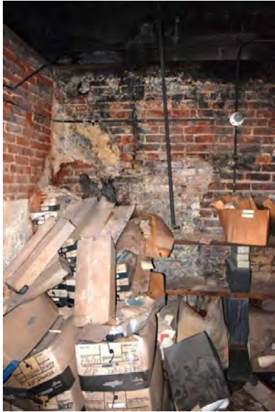
Figure 4.75: Brick foundation walls of old boiler room. Note current paper storage and moisture.
