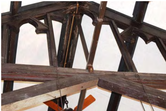
Figure 4.24: Longitudinal crack in collar tie
