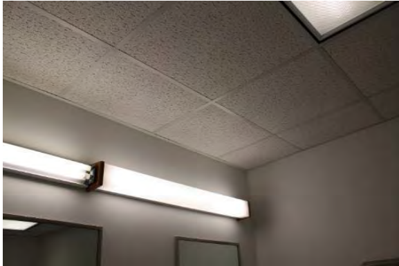
Figure 3.134, Historic Courthouse, Second Floor, Room 206, view of ceiling and lights above sink at the west wall; note the missing light cover at left.
