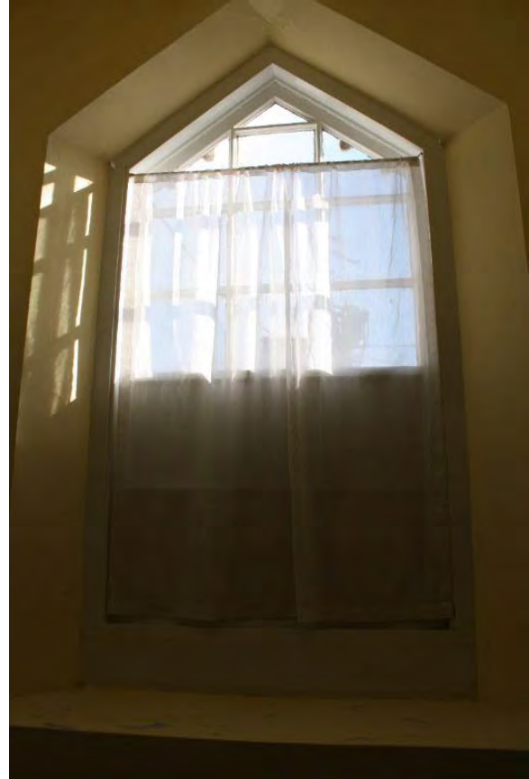
Figure 3.65, Historic Courthouse, First Floor, Room 114, view of window; the bottom panes are painted over.
