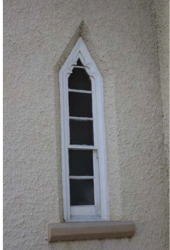
Figure 3.19, Historic Renwick Courthouse, north elevation, view of first-story lancet-shaped window at side wall of projecting gable end.
