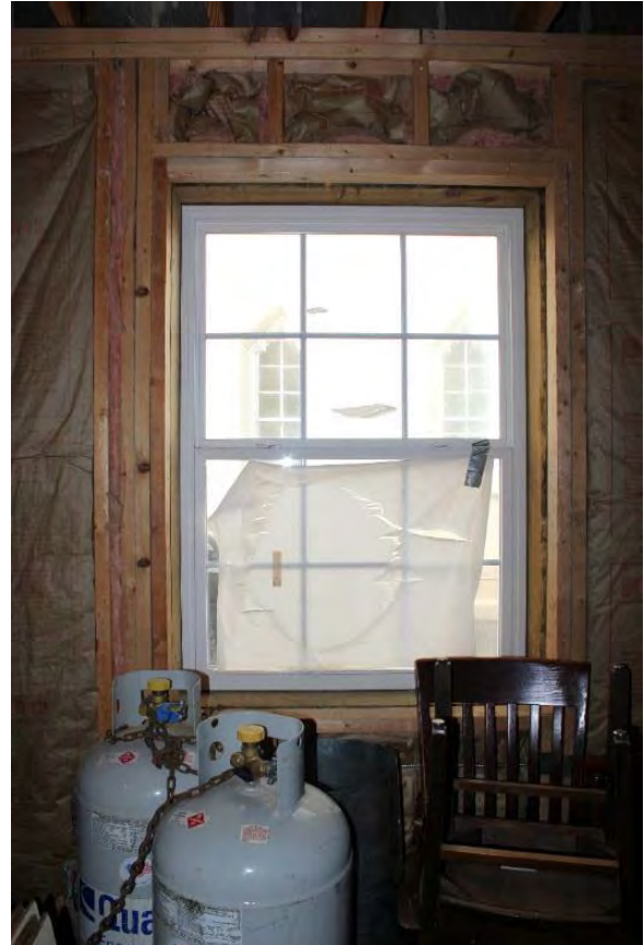
Figure 3.433, Old Jail, First Floor, Room 110, view of a vinyl replacement, six-over-six window at the west wall.
