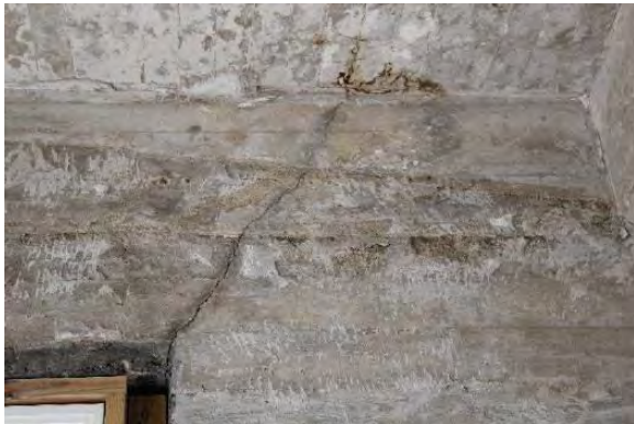
Figure 3.441, Old Jail, Second Floor, Room 201, view of a diagonal crack in the wall at the upper corner of the window.
