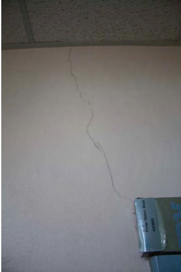
Figure 3.127, Historic Courthouse, Second Floor, Room 203, detail view of crack at the north wall.
