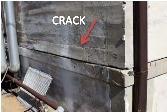
Figure 4.67: One-story extension with cracking and spalling concrete above the first floor slab edge
