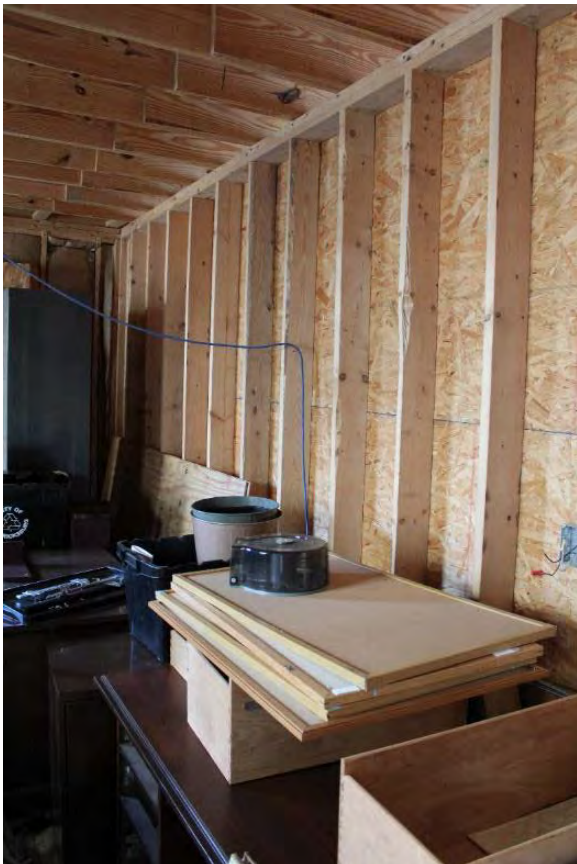
Figure 3.432, Old Jail, First Floor, Room 110, view of exposed framing and particle board at the east wall.
