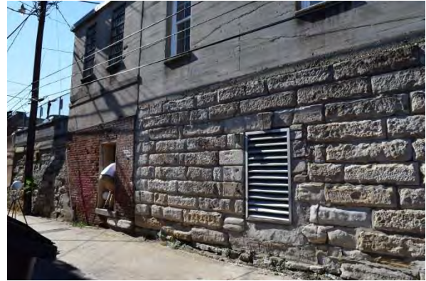
Figure 4.61: Historic brick and ashlar stone masonry foundation walls below more recent cast-in-place concrete structure above
