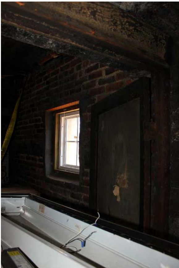
Figure 3.368, Old Jail, Basement, Room 003, view of the four-light, square, vinyl replacement window at the east wall and the adjacent interior door. Note the area of loss at the door.
