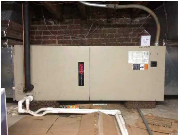
Figure 5.11: Library indoor unit, basement.
