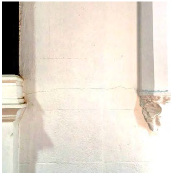
Figure 4.27: Cracking through plaster between window and truss pilasters.
