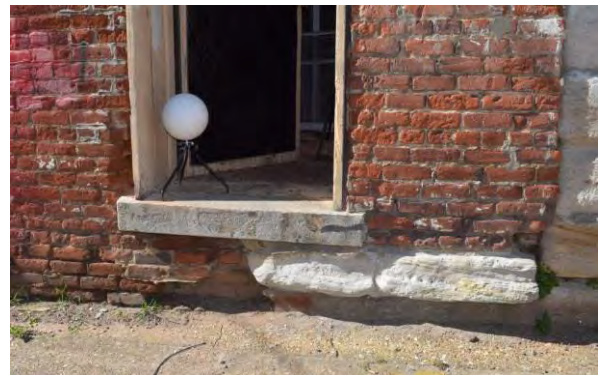
Figure 4.74: Loss of brick under threshold in foundation wall below 1-story extension
