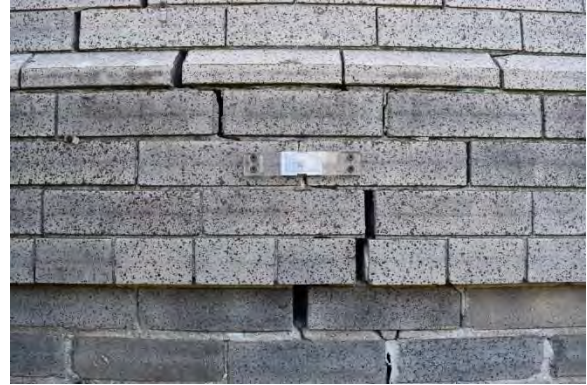
Figure 4.50: Abandoned crack monitoring
