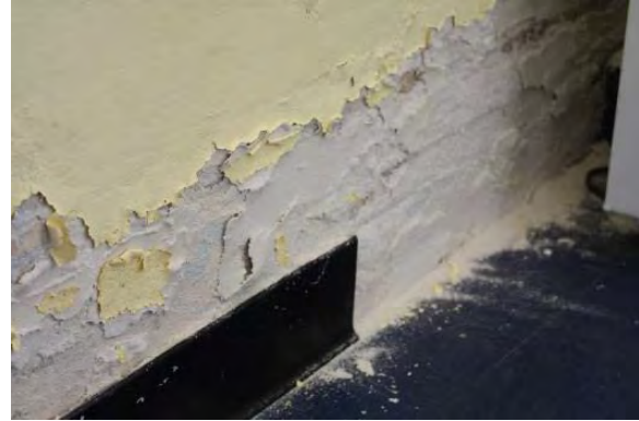
Figure 3.67, Historic Courthouse, First Floor, Room 115, view of damaged plaster and missing base at the east wall.
