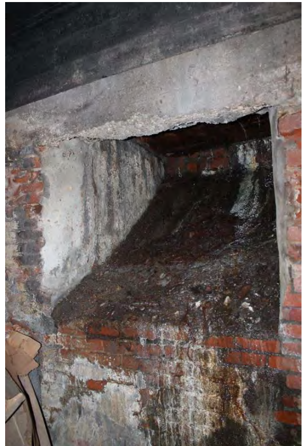
Figure 3.357, Old Jail, Basement, Room 001, view of the coal chute at the west wall. Note that the chute is heavily soiled and there is moisture staining at the wall below.
