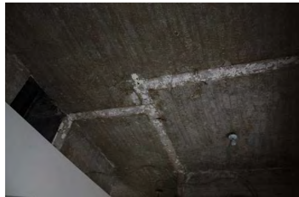
Figure 3.407, Old Jail, First Floor, Room 105, view of the poured-in-place concrete ceiling. Note the linear marks at the ceiling where there were formerly walls.
