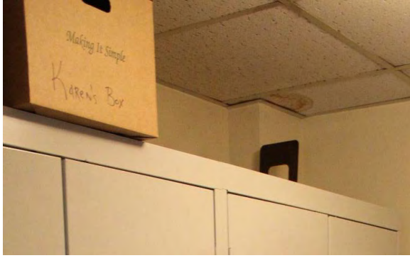
Figure 3.309, Old Wallace Library, Second Floor, Room 207, view of moisture staining at a ceiling tile.
