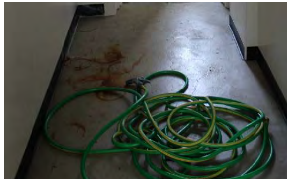
Figure 3.403, Old Jail, First Floor, Room 104, detail view of the circular rust stains at the floor in the center hall.
