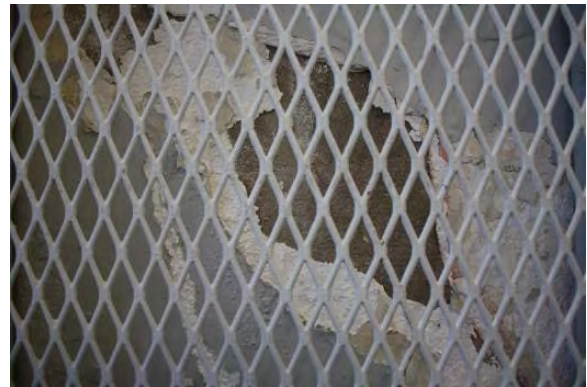
Figure 3.183, Historic Courthouse, Second Floor, Room 221, view of plaster damage due to efflorescence underneath the east window.
