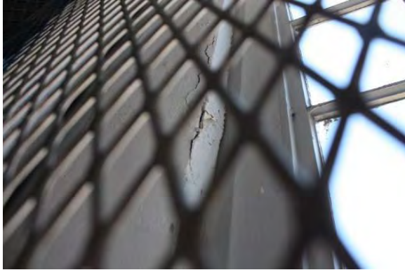
Figure 3.192, Historic Courthouse, Second Floor, Room 222, view of a crack at the reveal of the north window.
