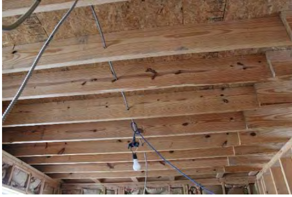
Figure 3.431, Old Jail, First Floor, Room 110, view of exposed wood floor framing at the ceiling.
