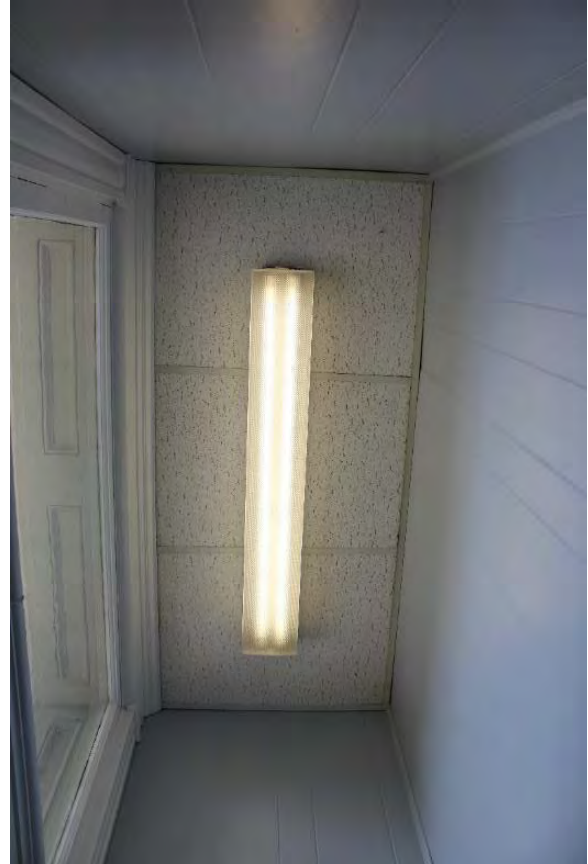
Figure 3.267, Old Wallace Library, First Floor, Room 102, view of suspended acoustical tile ceiling.
