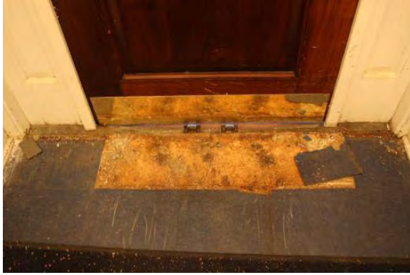
Figure 3.51, Historic Courthouse, First Floor, Room 103, view broken and missing floor tiles.
