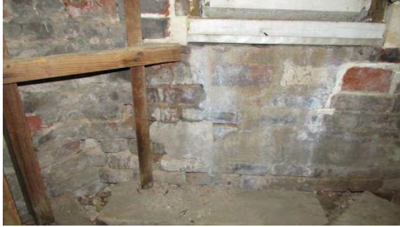
Figure 15: Masonry and wood deterioration just above the 3 rd floor level
