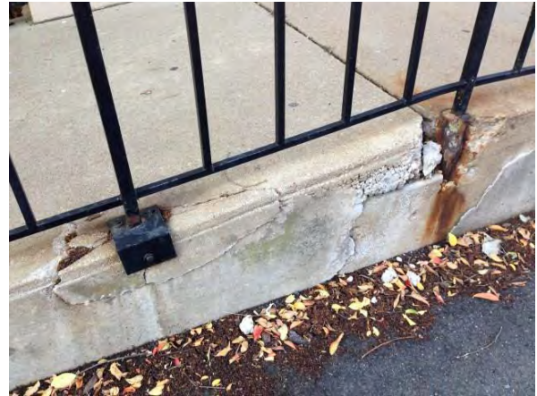
Figure 4.09: South entryway ramp with concrete spalling due to rusting railings
