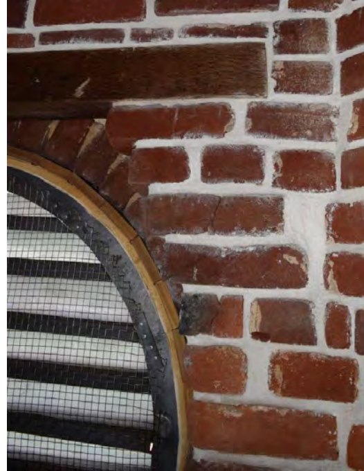
Figure 4.45: Cracking in corbelled brick jamb below wood lintel bearing
