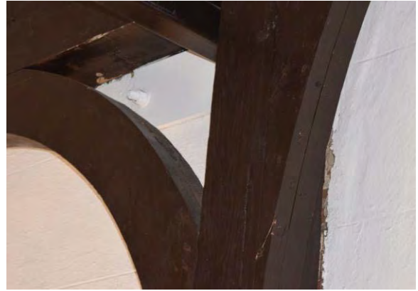
Figure 4.25: Transverse crack in collar brace
