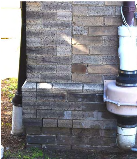
Figure 4.52: Open mortar joints at southwest corner
