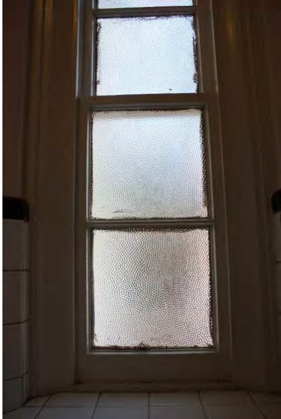
Figure 3.96, Historic Courthouse, First Floor, Room 124, view of the privacy glass at the lower sash of the window.
