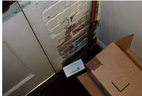
Figure 3.256, Old Wallace Library, Basement, Room 004, view of paint loss at east wall adjacent to the exterior door.
