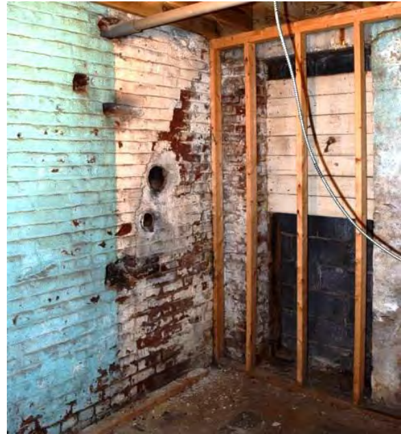
Figure 4.76: Brick foundation wall penetrations of northern jail addition. Note previous entrance to presumed tunnel with lintel distress.
