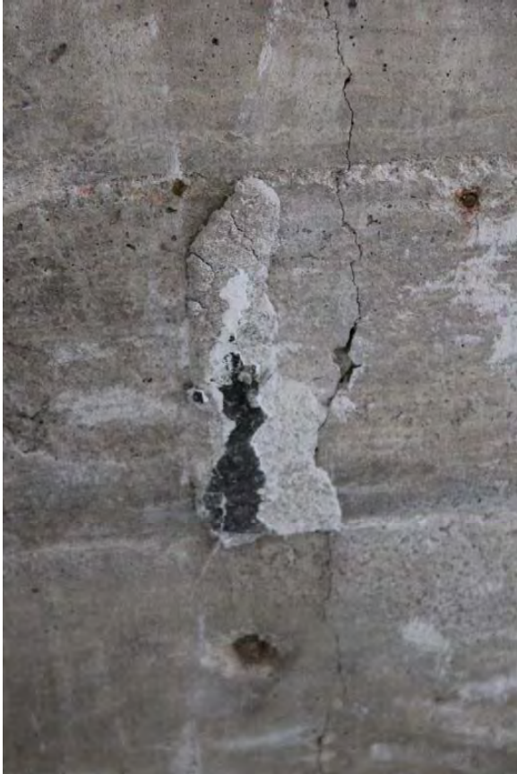
Figure 3.424, Old Jail, First Floor, Room 108, view of a crack in the wall at the stair hall.
