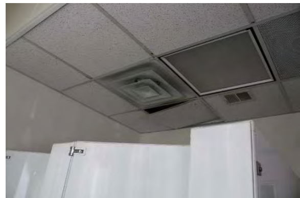
Figure 3.70, Historic Courthouse, First Floor, Room 116, view of the ceiling; note the displaced ceiling tile.
