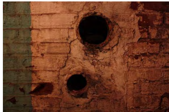
Figure 3.373, Old Jail, Basement, Room 004, detail view of holes at the south wall.
