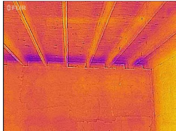
Figure 3.434A, Old Jail, First Floor, Room 111, infrared view of the joist ends. Note the cooler coloring where the joists intersect the exterior wall.
