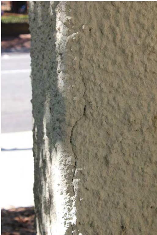
Figure 1.1, Renwick Courthouse, detail of exterior stucco. Note hairline cracks that result in moisture infiltration. Photograph 2015.
