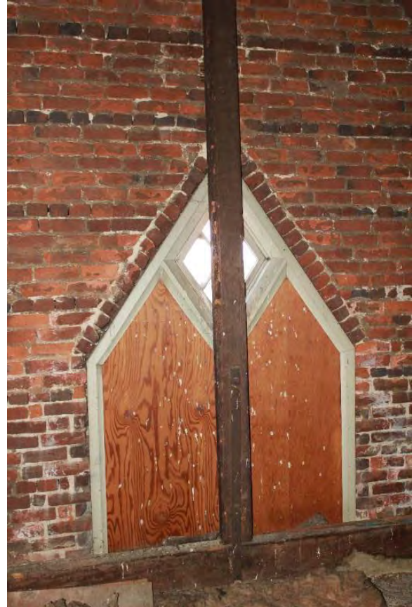
Figure 3.207, Historic Courthouse, North Attic, Room 303, view of east, center attic window. Note the boarded-up sashes.
