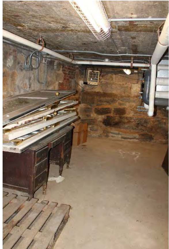
Figure 3.39, Historic Courthouse, Basement, Room 001, general view looking south. Note the deterioration of the concrete at the ceiling.
