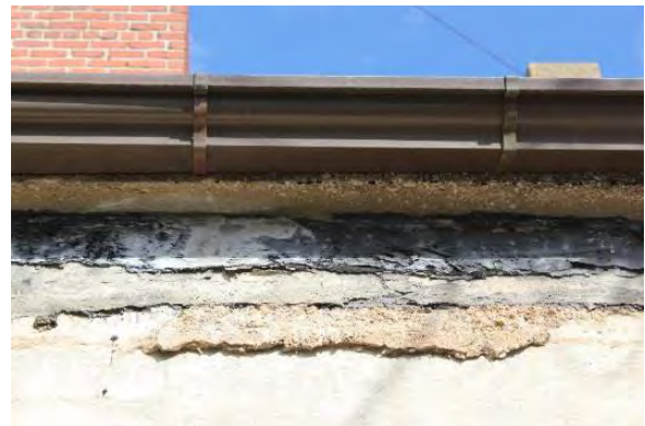
Figure 3.352, Old Jail, south elevation, view of spalling just below the cornice.
