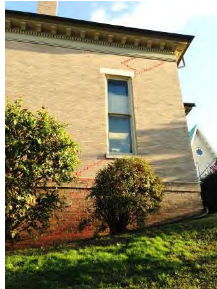
Figure 4.48: Diagonal cracking in North Façade
