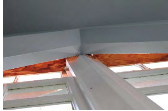
Figure 3.171, Historic Courthouse, Second Floor, Room 216, view of plywood between window and opening at head of center window at west wall.
