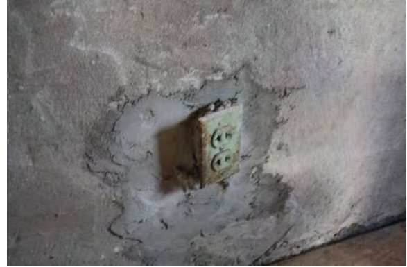
Figure 3.455, Old Jail, Second Floor, Room 202, view of a patch in the wall around an electrical outlet.
