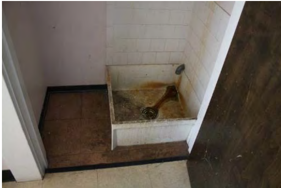
Figure 3.136, Historic Courthouse, Second Floor, Room 207, view of mop sink. Note heavy soiling and rust at both sink and tile and soiled floor.
