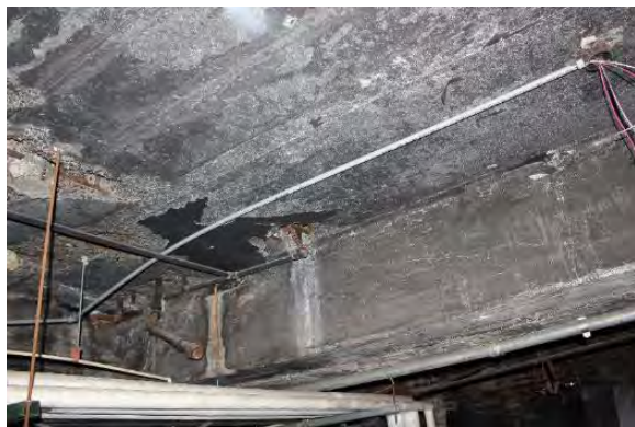
Figure 3.359, Old Jail, Basement, Room 002, view of poured-in-place concrete ceiling. Note the areas of loss and patching.
