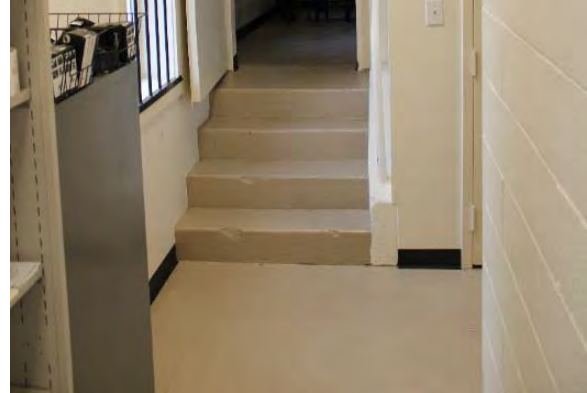
Figure 3.394, Old Jail, First Floor, Room 102, view of the concrete stair between Rooms 101 and 102. Note the small areas of loss at the ends of the treads.
