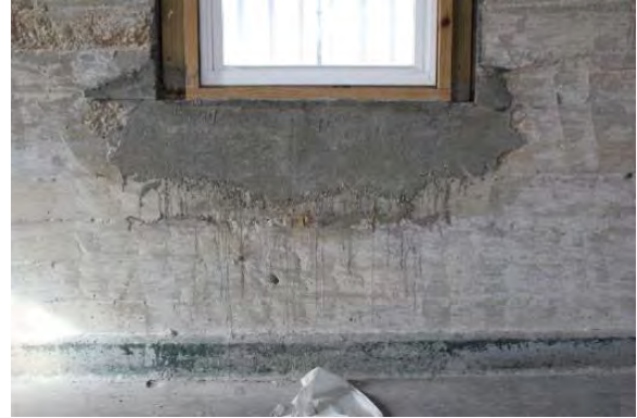
Figure 3.442, Old Jail, Second Floor, Room 201, view of a concrete patch under a window; similar patches are found at other windows.
