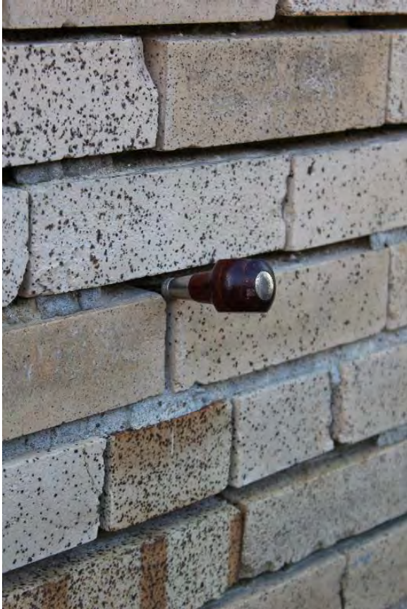
Figure 3.230, Wallace Library, East elevation, detail of brick wall. Note missing mortar.
