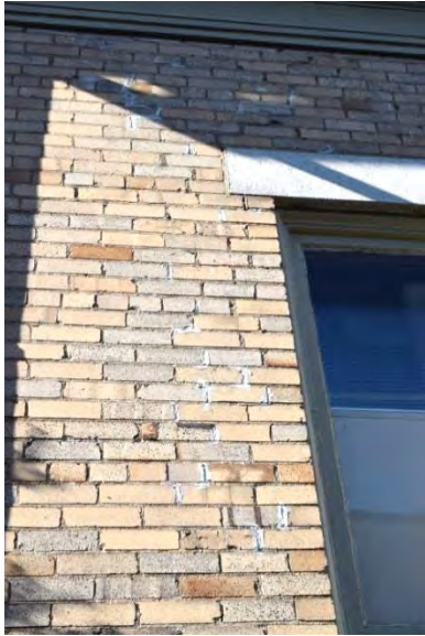
Figure 4.51: Incompatible repointing materials at south façade
