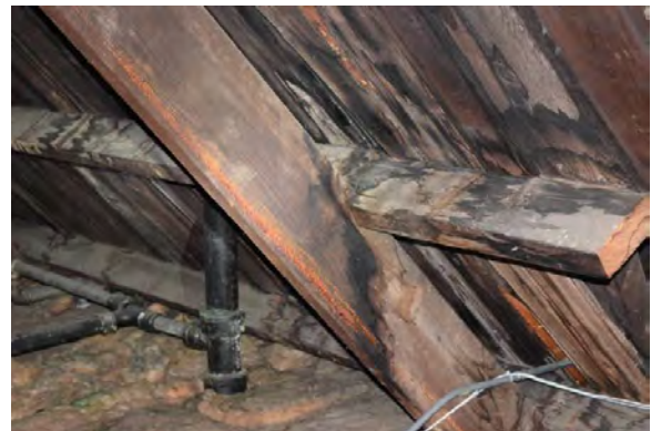
Figure 4.36: Water staining around opening of stairway opening
