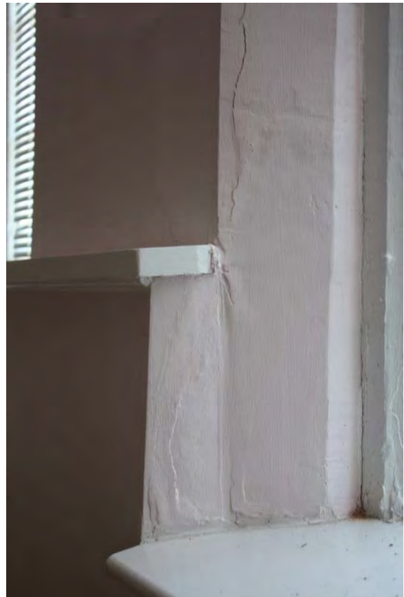
Figure 3.140, Historic Courthouse, Second Floor, Room 208, view of plaster damage at one of the window reveals.
