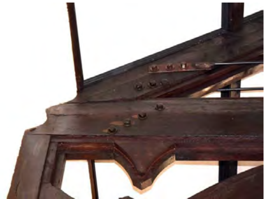
Figure 4.26: Crushing of hammer beam end and localized cracking at tie rod connection to top chord.
