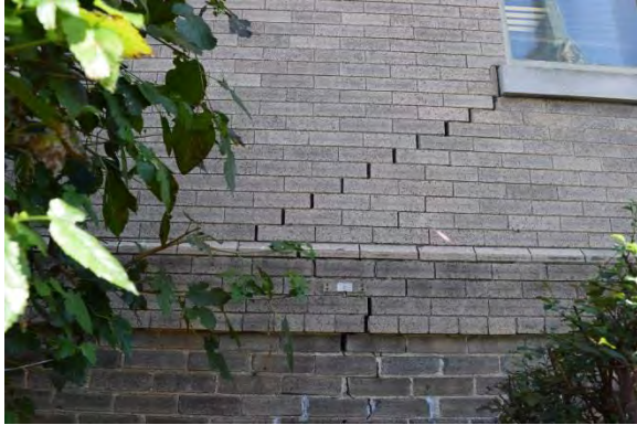
Figure 4.49: Diagonal cracking in North Façade
