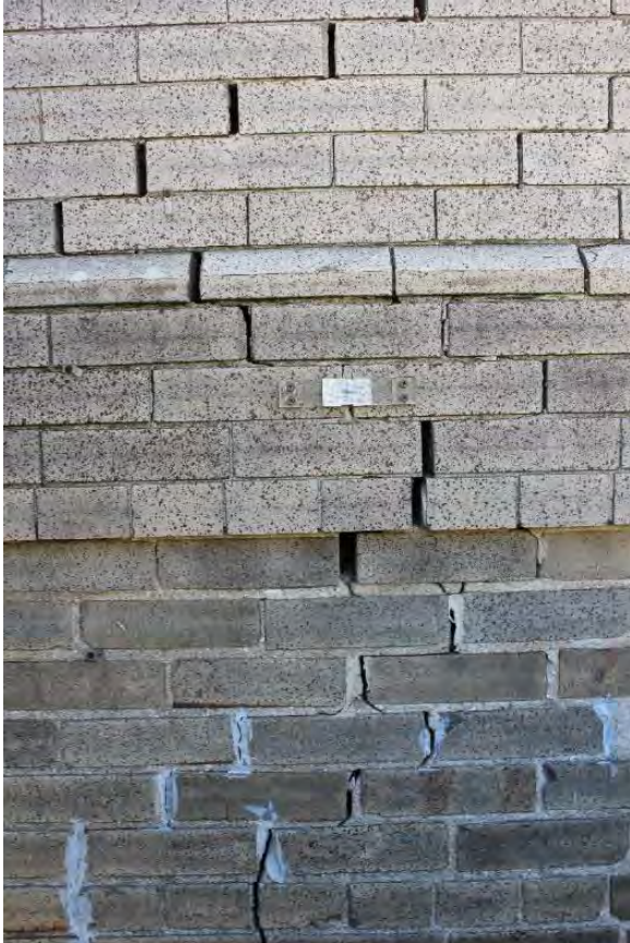
Figure 3.225, Wallace Library, North elevation, detail crack and shifting damage.
