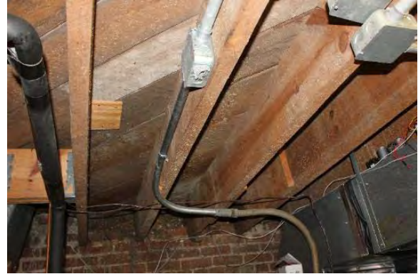
Figure 3.246, Old Wallace Library, Basement, Room 001, view of exposed floor framing of the first floor above.
