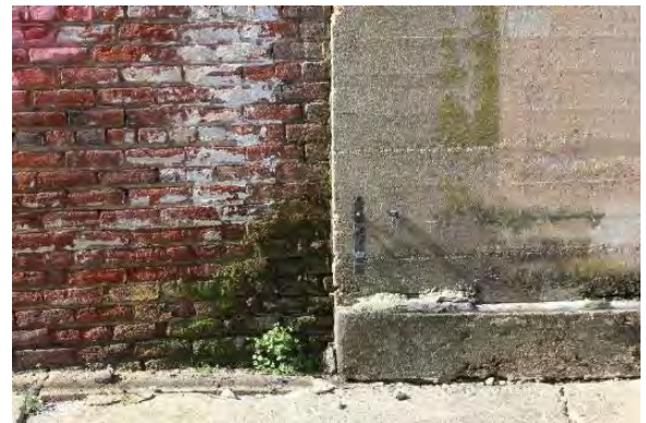
Figure 3.339, Old Jail, east elevation, view of basement at intersection of high- and low-roofed sections at the north end of the building. Note the large area of biological growth.
