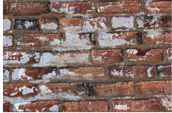
Figure 3.342, Old Jail, east elevation, detail view of brick at basement level of center section; note the efflorescence.
