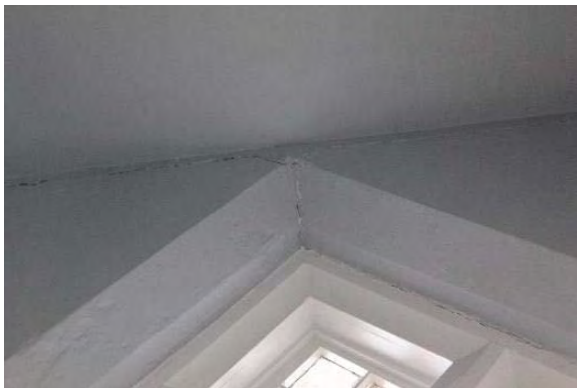
Figure 3.167, Historic Courthouse, Second Floor, Room 216, view of crack at head of window at north wall.
