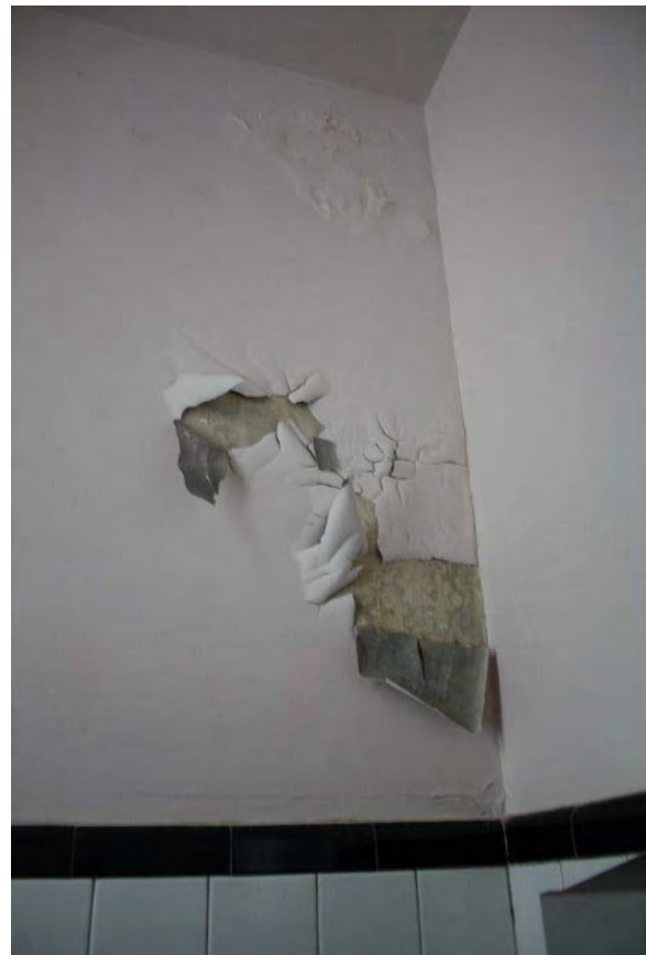
Figure 3.95, Historic Courthouse, First Floor, Room 124, view of damage to the plaster and paint at the north wall near the northeast corner of the room.
