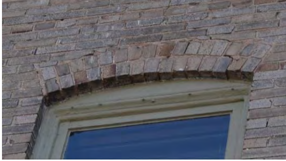
Figure 4.55: Brick displacement and joint cracks at segmental arch in east facade of Wallace Library
