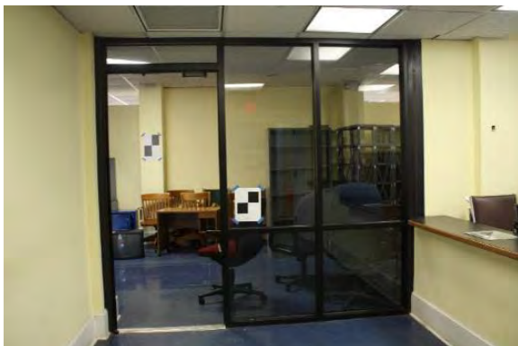
Figure 3.77, Historic Courthouse, First Floor, Room 118, view looking east at the storefront windows; note the missing door at left.
