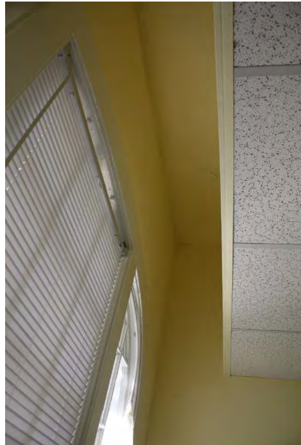
Figure 3.53, Historic Courthouse, First Floor, Room 105, view of high plaster ceiling and suspended acoustical tile ceiling.
