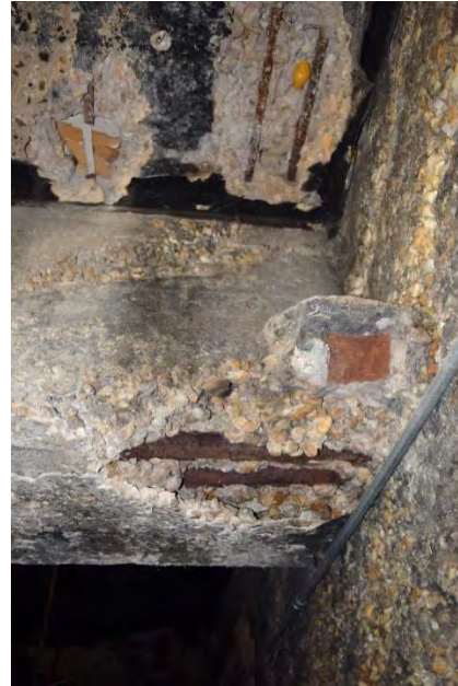
Figure 4.77: Beam 1 and exposed reinforcing
