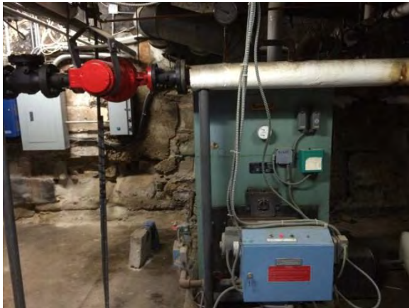
Figure 5.1: Boiler in Old Jail Basement
