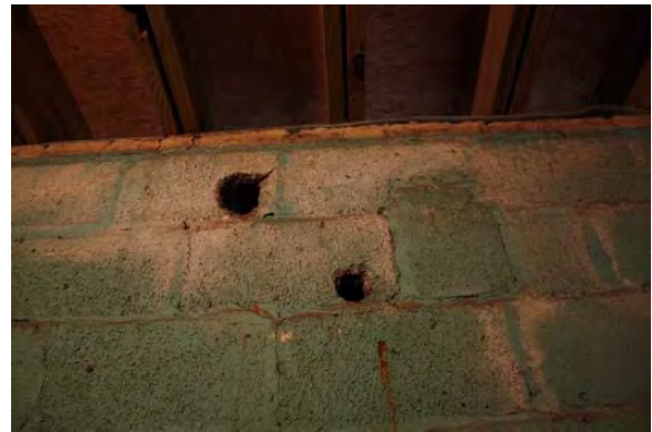
Figure 3.379, Old Jail, Basement, Room 005, detail view of holes at the east wall.
