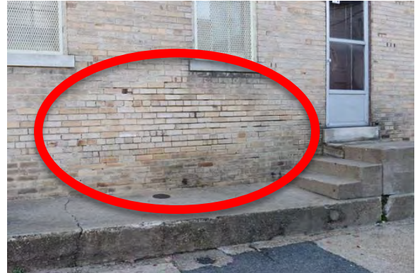
Figure 4.53: East façade with water infiltration
