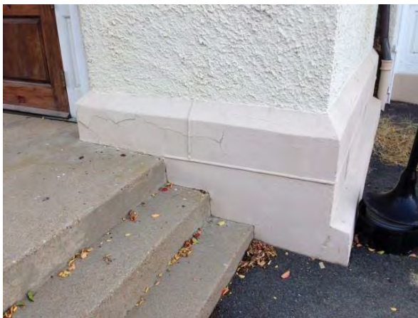
Figure 4.08: North stair to courthouse with crack in stucco near base.
