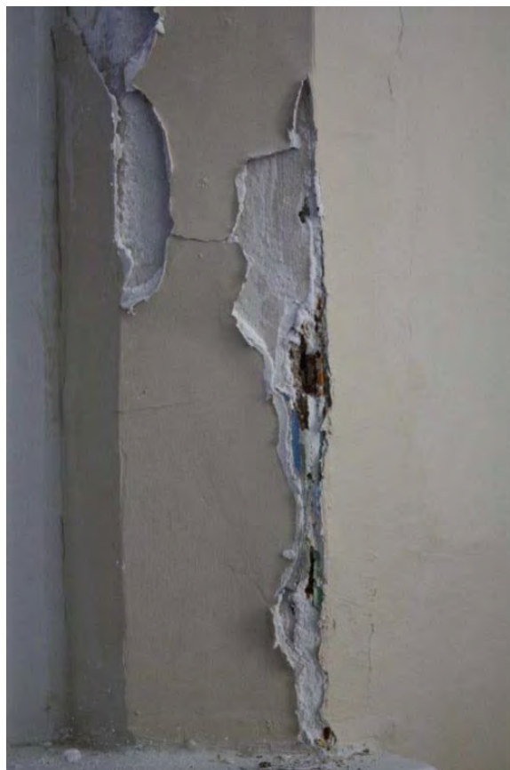
Figure 3.102, Historic Courthouse, First Floor, Room 127, view of plaster damage and efflorescence at the reveal of the easternmost window at the north wall.
