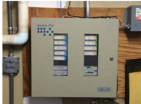
Figure 5.3: Building Automation System, Siemens 600 model.
