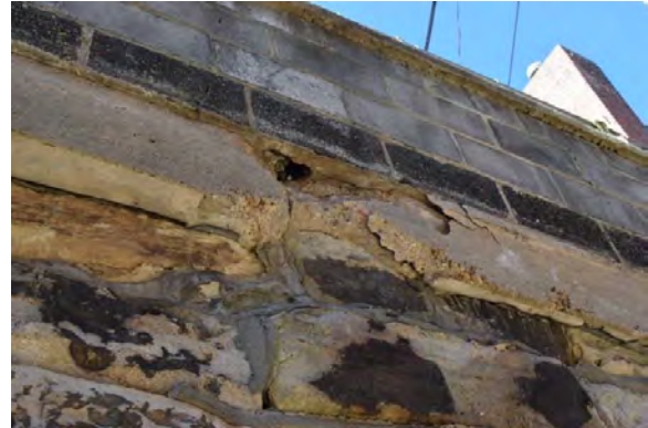
Figure 4.71: Cracked and spalling concrete at southeast retaining wall below parking lot
