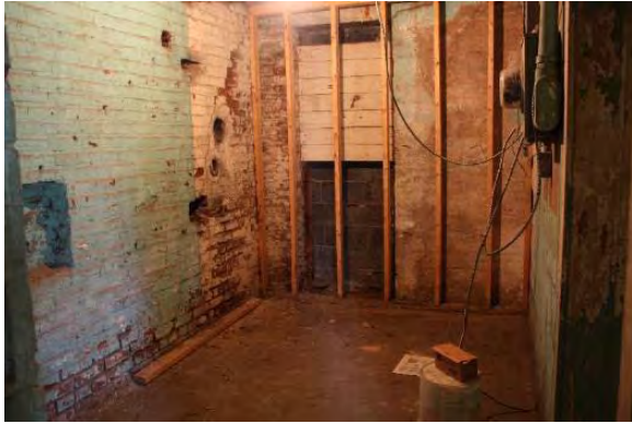
Figure 3.370, Old Jail, Basement, Room 004, general view looking west. Note the holes at the south wall; the former door opening infilled with concrete block; the large areas of paint loss; and the mix of building materials at the walls.
