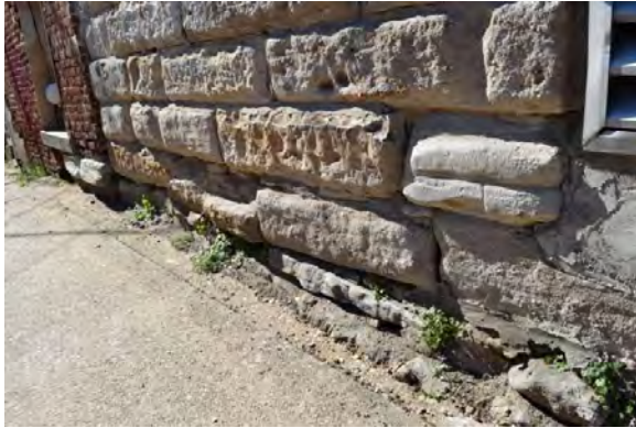
Figure 4.72: Early stone foundation wall under central portion of jail building. Note corner of louver on right.
