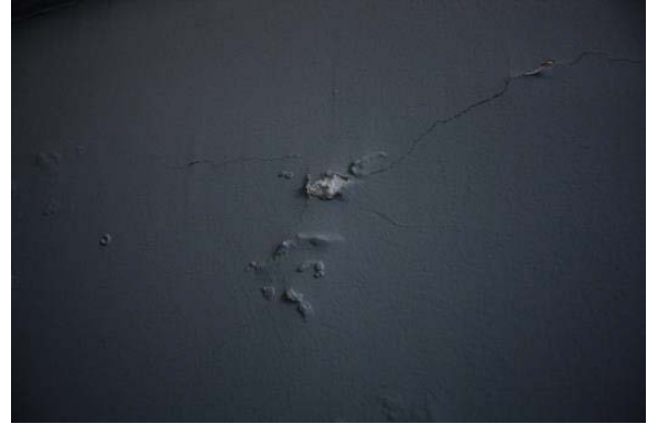
Figure 3.168, Historic Courthouse, Second Floor, Room 216, view of efflorescence below center window at west wall.
