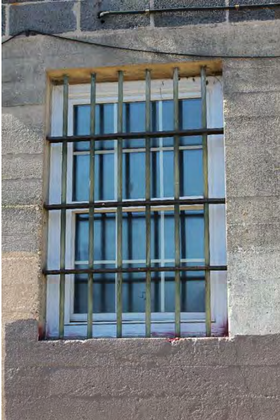
Figure 3.343, Old Jail, east elevation, view of one of the vinyl replacement windows at the basement level of the main, high-roofed section.
