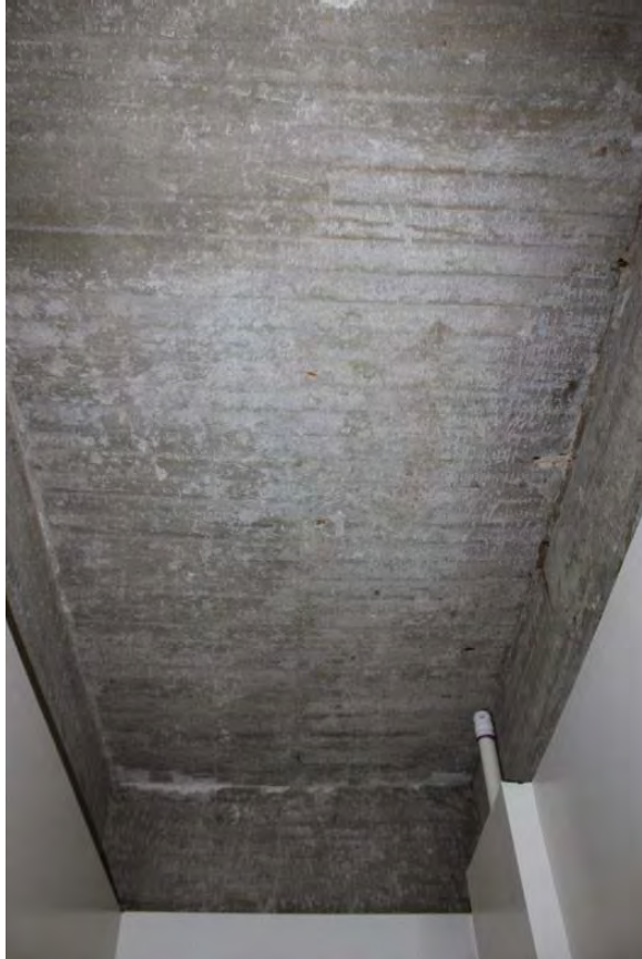
Figure 3.401, Old Jail, First Floor, Room 104, view of poured-in-place concrete ceiling at the center hall. Note that the concrete continues along the top edges of the walls.
