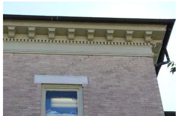
Figure 3.224, Wallace Library, North elevation, detail of cornice. Note the stepped cracks above the window.
