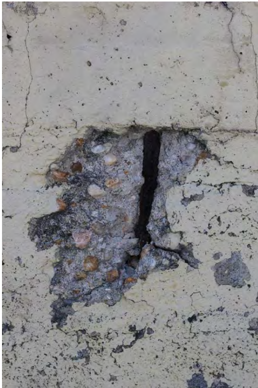
Figure 1.15, Old Jail. Rust-jacking and spalling of the exterior concrete wall surfaces. Photograph 2015.
