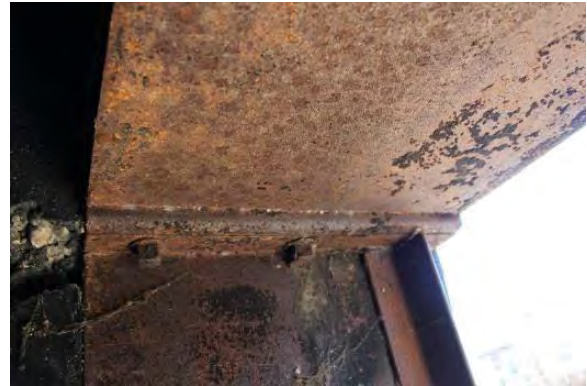
Figure 3.369, Old Jail, Basement, Room 003, view of the rusted frame of the exterior door at the east wall.
