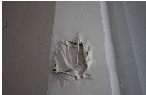
Figure 3.114, Historic Courthouse, First Floor, Room 132 (Stairway 2), view of paint failure due to moisture at the reveal of the window at the east wall.
