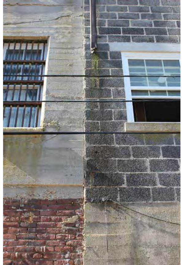
Figure 3.338, Old Jail, east elevation, view of intersection of high- and low-roofed sections at the north end of the building. Note the mix of building materials and the damaged, truncated downspout.
