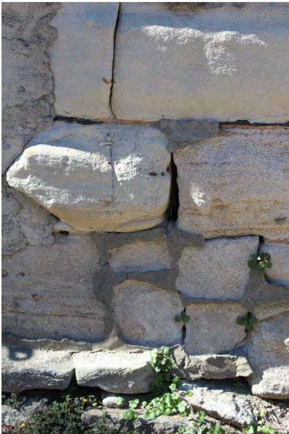
Figure 3.341, Old Jail, east elevation, detail view of rustic masonry at basement level; note the large areas of mortar loss.
