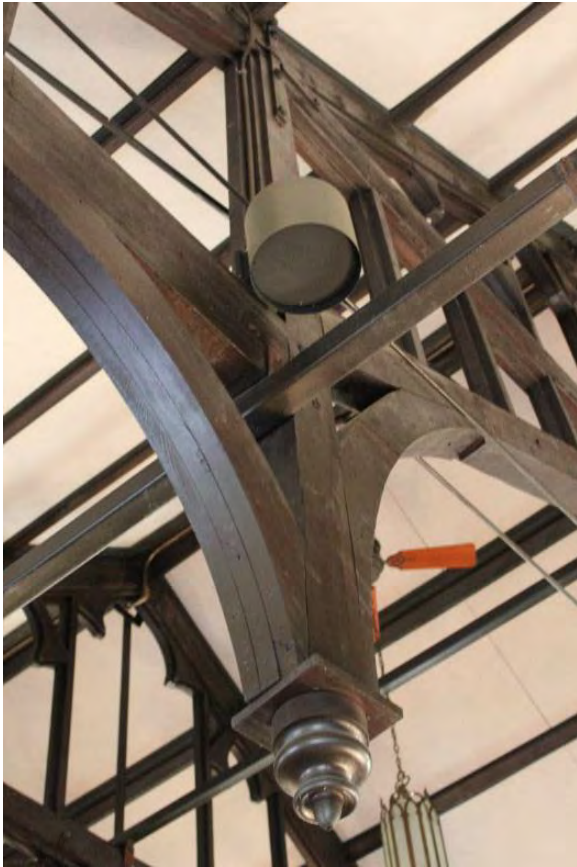
Figure 3.149, Historic Courthouse, Second Floor, Room 212, view of a pendant descending from one of the trusses.
