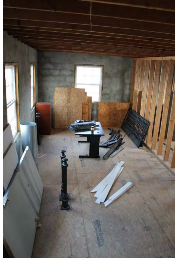
Figure 3.452, Old Jail, Second Floor, Room 202, general view looking north in the west end of the room.
