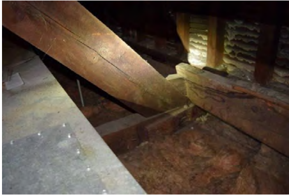
Figure 4.17: Crushing truss bearing end
