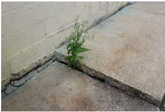
Figure 3.331, Old Jail, west elevation, view of uneven concrete walk.
