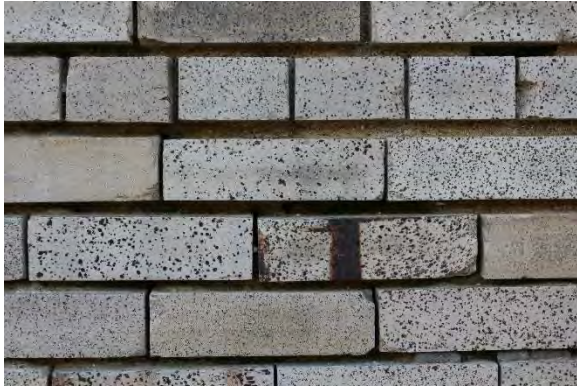
Figure 1.9, Wallace Library. Extensive mortar loss in the north elevation. Photograph 2015.
