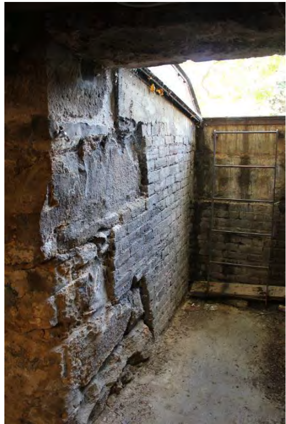
Figure 3.42, Historic Courthouse, Basement, Room 001, view of vestibule at north wall and underside of bulkhead door. Also note the transition from rubble stone walls to brick.
