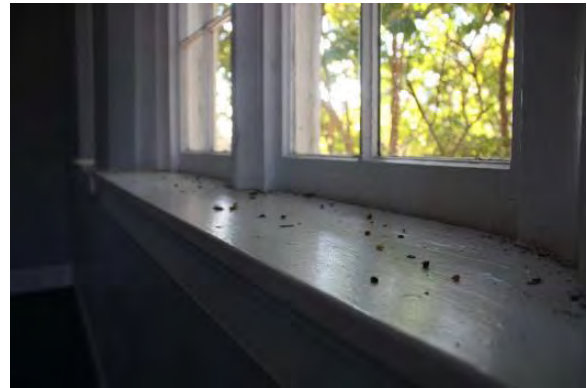
Figure 3.172, Historic Courthouse, Second Floor, Room 216, view of dead insects at sill of center window of west wall.
