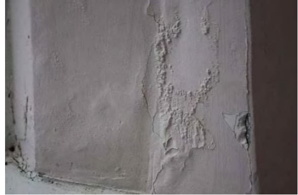
Figure 3.139, Historic Courthouse, Second Floor, Room 208, view of plaster damage at one of the window reveals.
