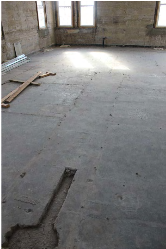
Figure 3.450, Old Jail, Second Floor, Room 201, view of scarring at the floor from former jail cell walls and sanitary line.
