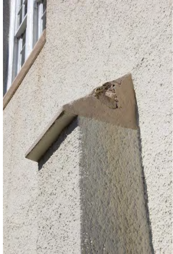
Figure 3.32, Historic Renwick Courthouse, south elevation, detail view of stucco buttress with stone amortizement. Note the damaged amortizement.
