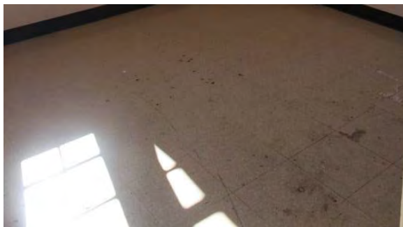
Figure 3.145, Historic Courthouse, Second Floor, Room 209, view of soiling and scuffing at floor.
