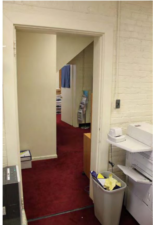
Figure 3.254, Old Wallace Library, Basement, Room 003, view of doorway at south wall; note remnants of hinges at trim, indicating that a door has been removed.
