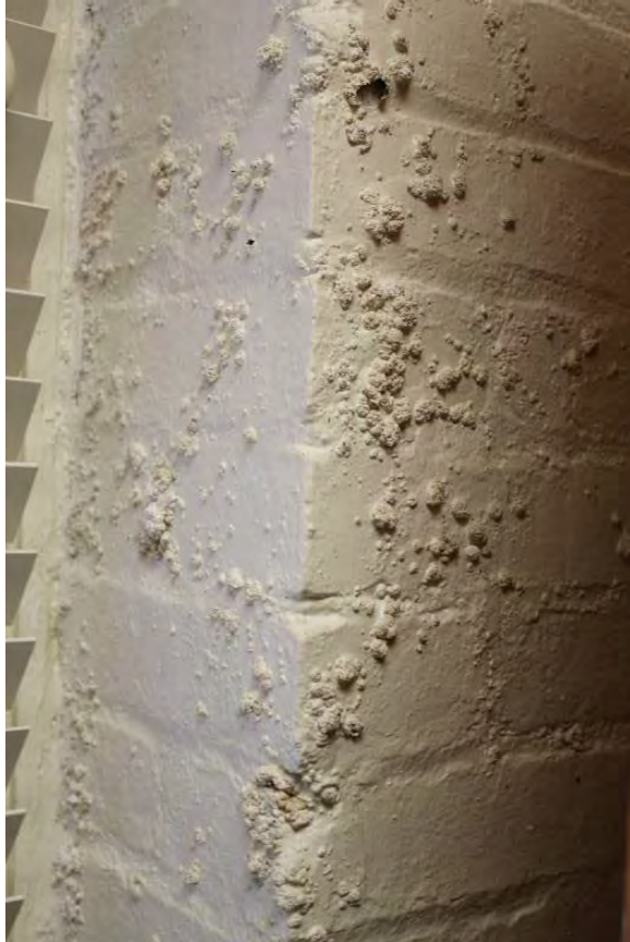
Figure 3.262, Old Wallace Library, Basement, Room 005, additional view of efflorescence adjacent to the south window.
