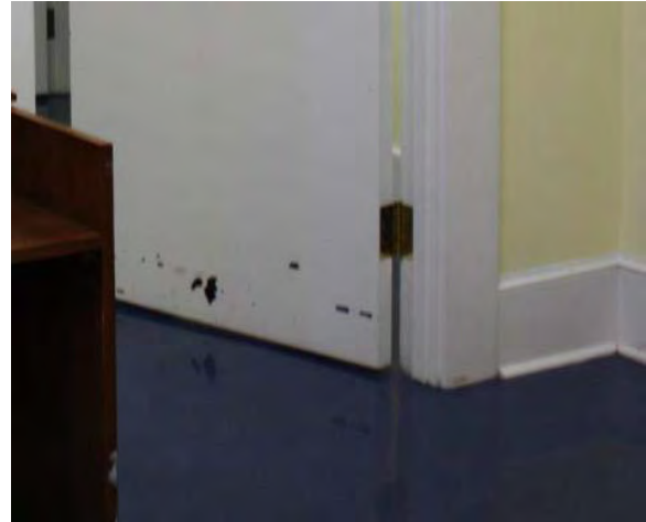
Figure 3.85, Historic Courthouse, First Floor, Room 120, view of paint loss at the base of the north door.
