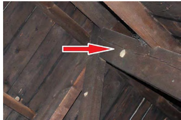
Figure 4.16: shear crack in top chord of north wing king post roof trusses
