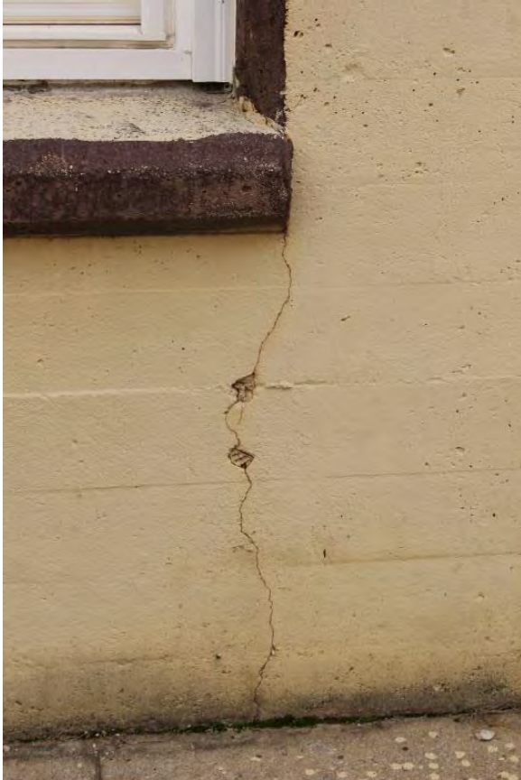
Figure 3.324, Old Jail, west elevation, view of a crack underneath the first-story window south of the northernmost door.
