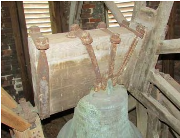
Figure 7: Yoke timber and iron for bell support
