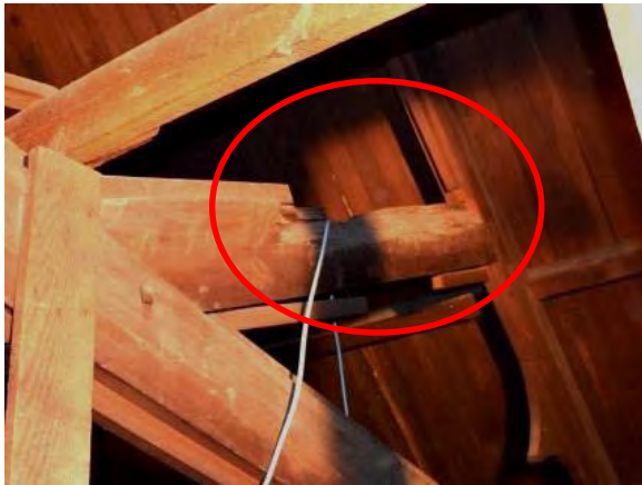
Figure 4.38: Deteriorated scissor truss brace in south wing
