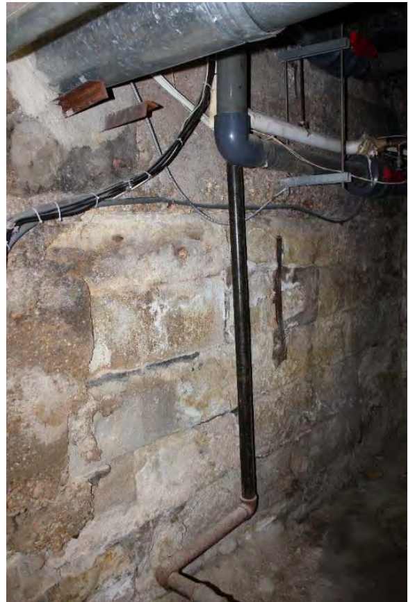
Figure 3.360, Old Jail, Basement, Room 002, view of efflorescence at stone walls.
