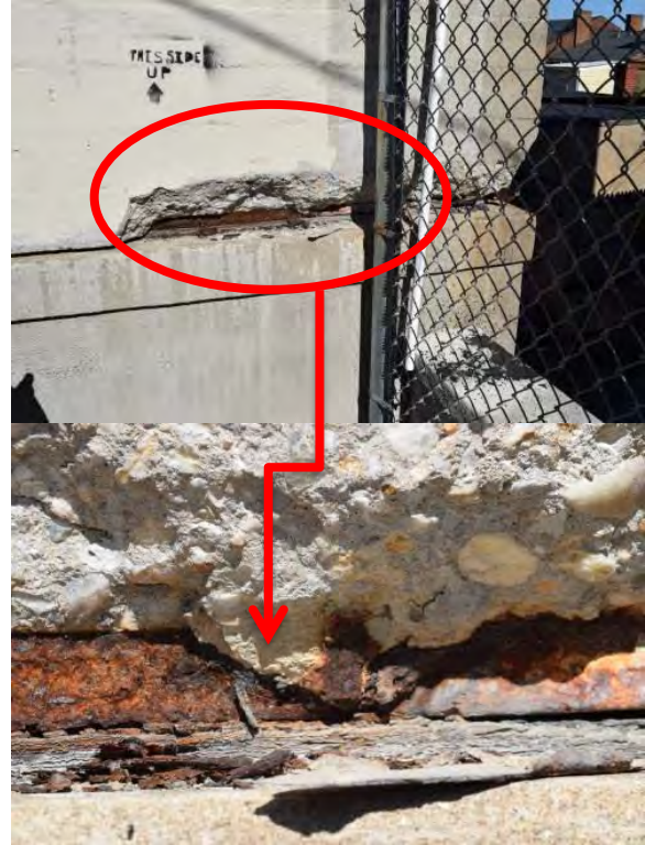
Figure 4.68: Spalling concrete and delaminated steel at southeast corner of jail
