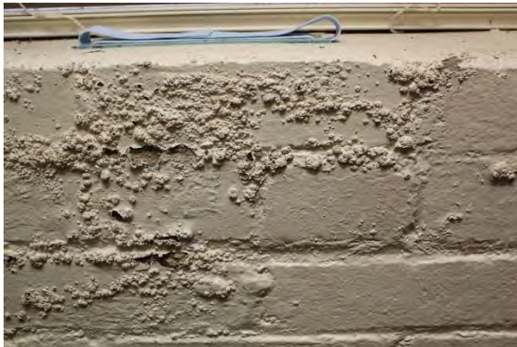
Figure 1.10, Wallace Library. Persistent moisture infiltration in the basement. Photograph 2015.
