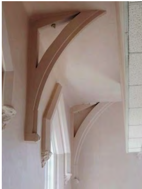
Figure 4.34: South wing scissor truss ends below 2 nd floor ceiling. Note two layers of ceiling.
