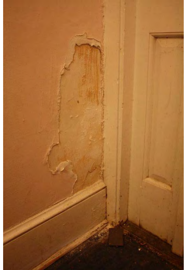
Figure 3.50, Historic Courthouse, First Floor, Room 102, view of efflorescence at the plaster walls near the exterior door.
