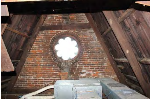
Figure 3.208, Historic Courthouse, North Attic, Room 303, view of round, multi-foil window at north gable end.
