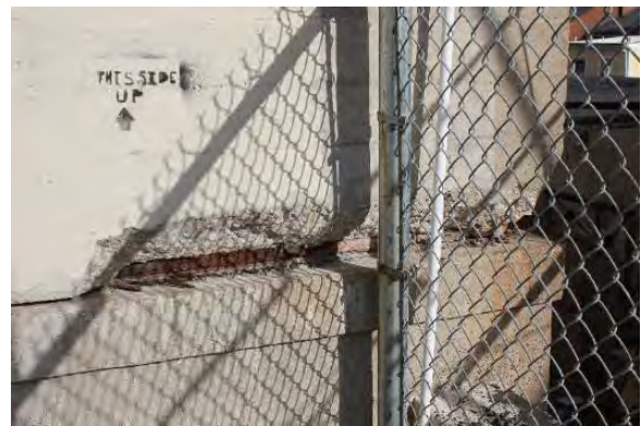
Figure 3.351, Old Jail, south elevation, view of an area of loss in the concrete wall at the southeast corner of the one-story wing.
