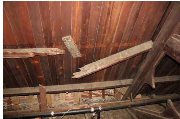
Figure 1.3, Fredericksburg Courthouse, North attic. Broken truss. Photograph 2015.
