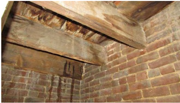
Figure 22: 2 nd floor joist bearing deterioration
