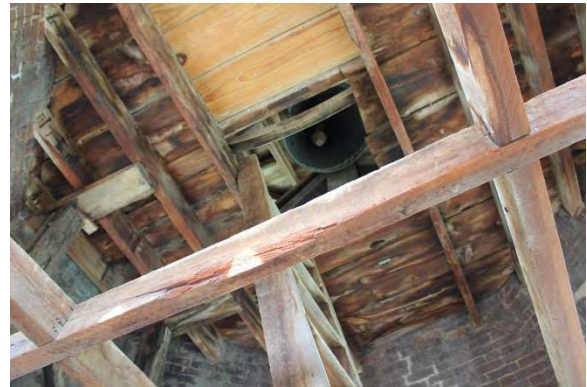
Figure 1.4, Fredericksburg Courthouse, bell tower. Moisture infiltration into the bell tower. Photograph 2015.
