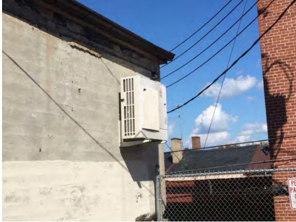
Figure 5.19: Jail, mini-split condensing unit.
