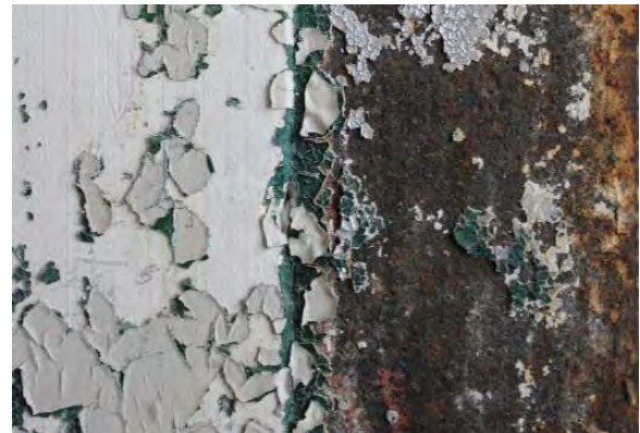
Figure 3.446, Old Jail, Second Floor, Room 201, view of heavy rust and paint loss at the east jail cell door's metal trim, a condition also found at the trim of the west doorway trim.
