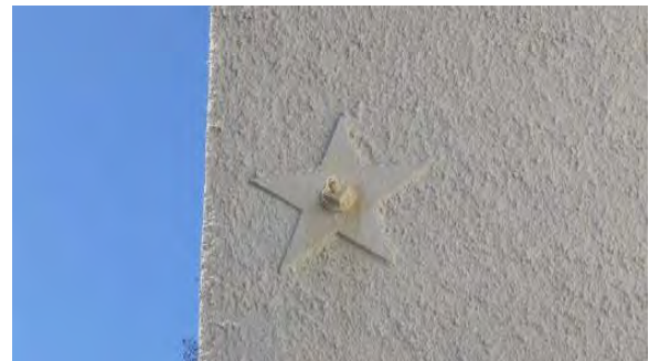
Figure 3.33, Historic Renwick Courthouse, south elevation, detail view of star-shaped tie rod at side wall of projecting gable end.
