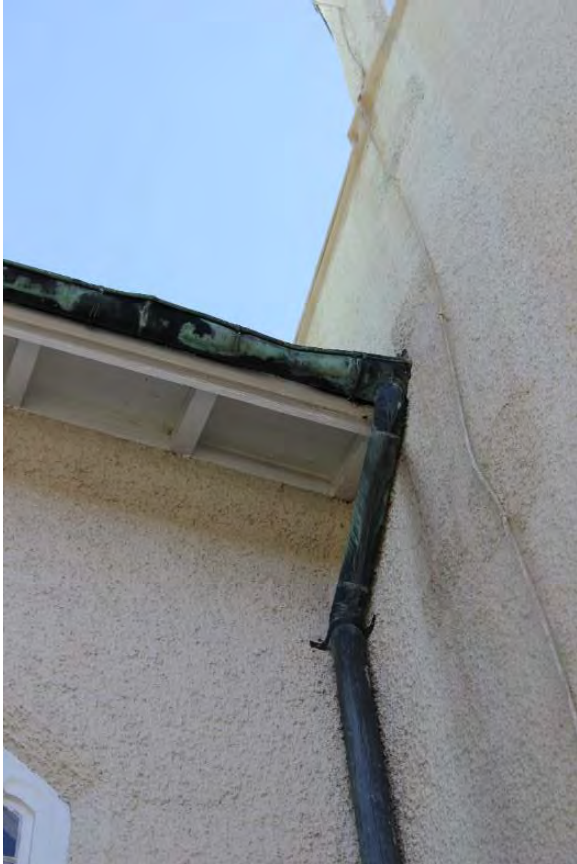
Figure 3.17, Historic Renwick Courthouse, north elevation, view of round copper gutter and downspout.
