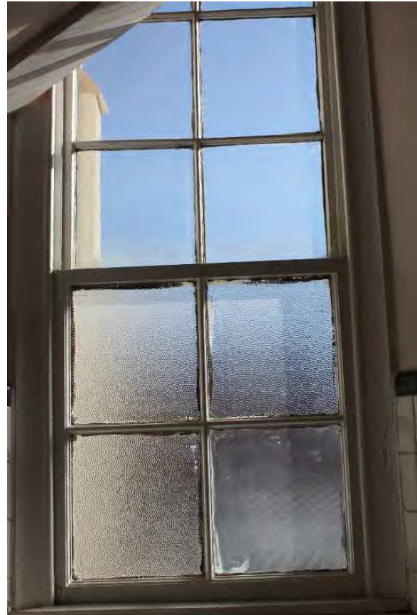
Figure 3.48, Historic Courthouse, First Floor, Room 102, view of window with privacy glass and stray paint at the panes.
