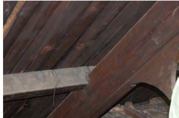
Figure 4.32: Purlins notched above truss top chord. Note purlins are discontinuous.
