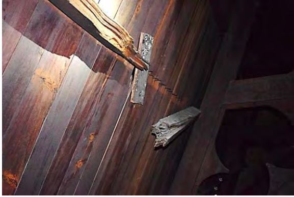
Figure 4.37: Broken purlin at center bay of trusses
