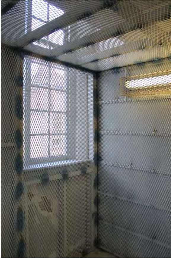
Figure 3.181, Historic Courthouse, Second Floor, Room 221, general view looking southeast. Note the area of plaster damage under the window.
