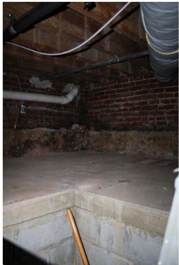
Figure 3.247, Old Wallace Library, Basement, Room 001, view of the concrete block ledge at the southwest corner of the room; note the biological growth where the ledge meets the wall.
