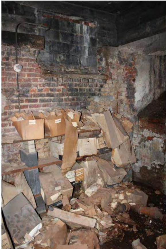
Figure 3.354, Old Jail, Basement, Room 001, general view looking southwest. Note the many moisture-deteriorated cardboard boxes and papers stored in the room and moisture staining under the infilled window.
