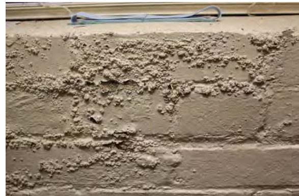
Figure 3.261, Old Wallace Library, Basement, Room 005, view of efflorescence at the painted brick wall underneath the south window.
