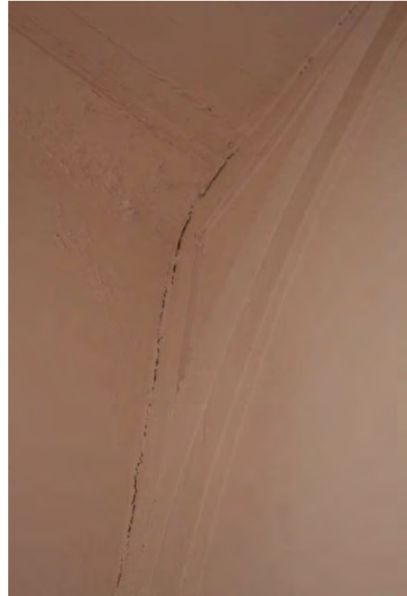
Figure 3.143, Historic Courthouse, Second Floor, Room 211, view of west brace separating from the wall.
