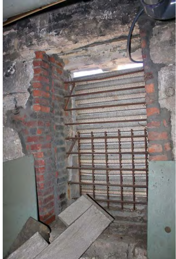
Figure 3.362, Old Jail, Basement, Room 003, view of a mechanical grille and metal bars at the east wall; note that the bars are rusted.
