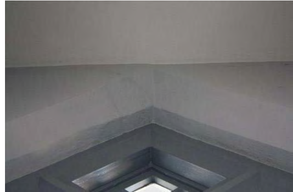
Figure 3.179, Historic Courthouse, Second Floor, Room 219, view of water damage at head of window.
