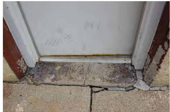
Figure 3.330, Old Jail, west elevation, view of cracked concrete at threshold of south door.
