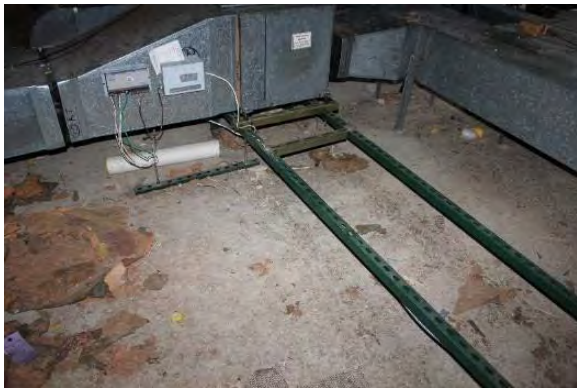
Figure 3.209, Historic Courthouse, North Attic, Room 303, view of concrete floor and air ducts.
