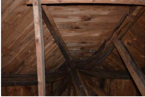
Figure 4.46: Cupola framing with water deterioration
