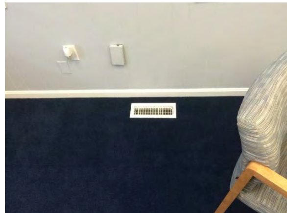
Figure 5.14: Library floor diffuser, first floor.
