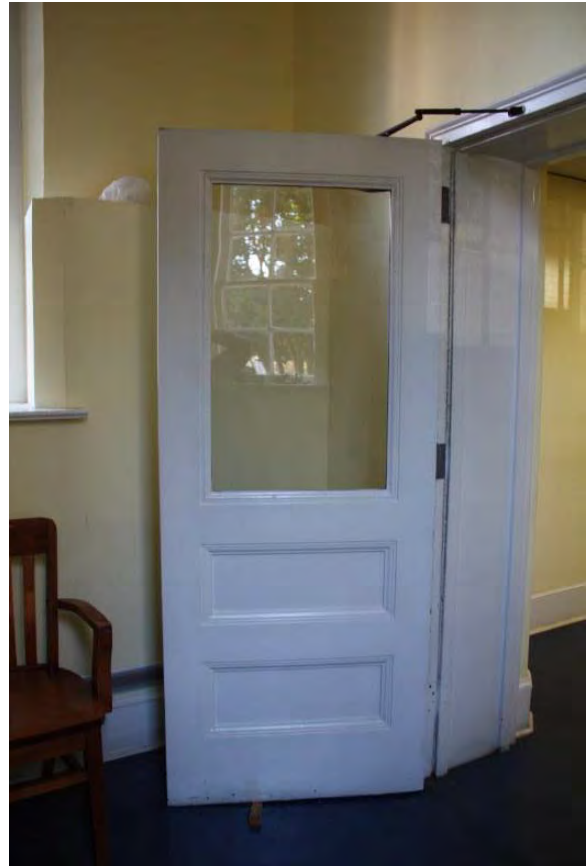
Figure 3.83, Historic Courthouse, First Floor, Room 119, view of one of paneled wood doors at the east wall.
