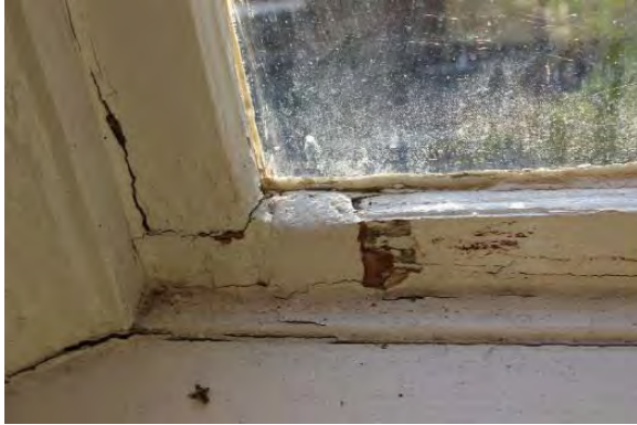
Figure 3.125, Historic Courthouse, Second Floor, Room 202, view of wood deterioration and cracking at a window frame.
