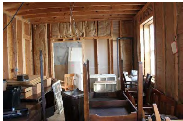
Figure 3.430, Old Jail, First Floor, Room 110, general view looking south. Note the unfinished state of the room and the large quantity of stored furniture and other materials.
