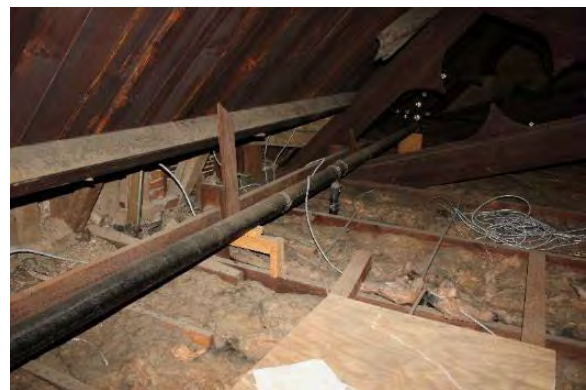
Figure 3.200, Historic Courthouse, South Attic, Room 301, view of attic floor and exposed pipes.
