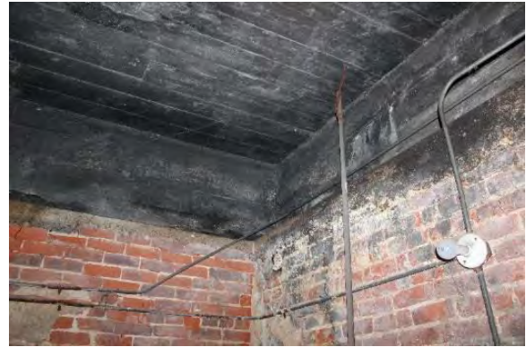
Figure 3.355, Old Jail, Basement, Room 001, view of efflorescence at the south brick wall.
