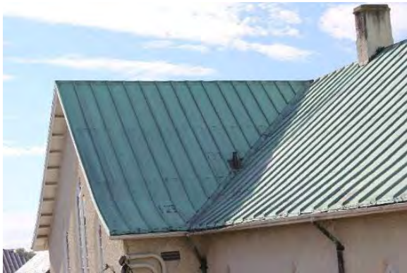
Figure 3.23, Historic Renwick Courthouse, east elevation, view of the standing-seam copper gable roof at the north crossing gable.
