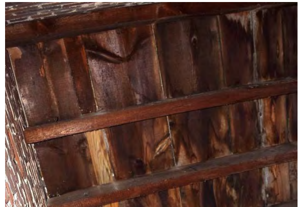
Figure 4.43: Wood bearing ends with water damage at 2 nd floor framing level
