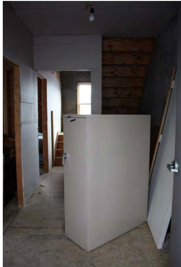
Figure 3.425, Old Jail, First Floor, Room 109, general view looking east. Note the unfinished state of the room.
