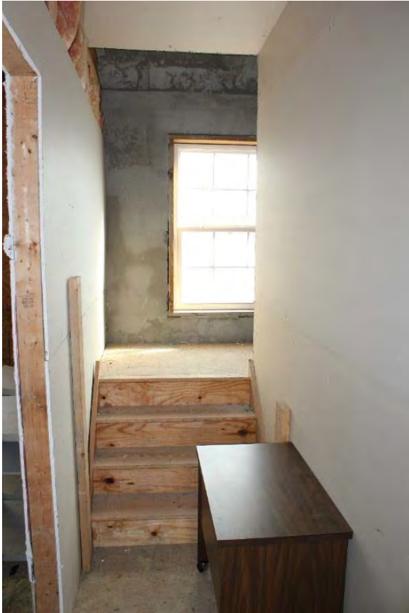
Figure 3.428, Old Jail, First Floor, Room 109, view looking east at the lower flight of stairs and the landing.
