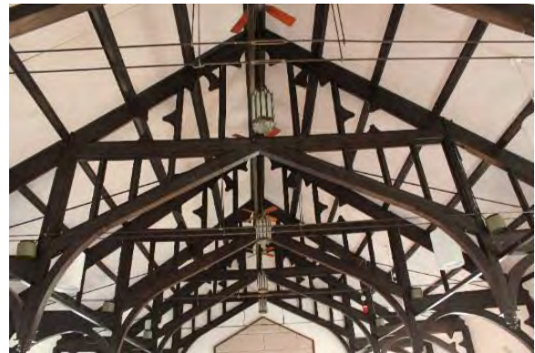
Figure 3.148, Historic Courthouse, Second Floor, Room 212, view of the Gothic Revival-style hammer beam trusses and acoustic paneling at the ceiling.
