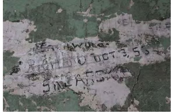
Figure 3.412, Old Jail, First Floor, Room 106, view of graffiti at the wall.
