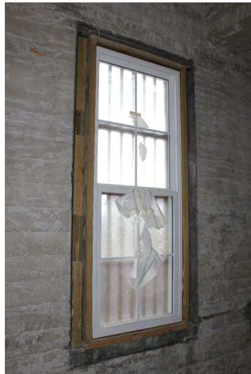
Figure 1.17, Old Jail. Nonfunctional window. Photograph 2015.
