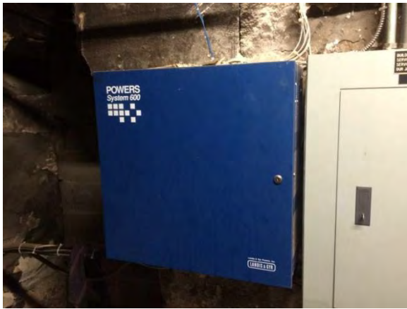
Figure 5.4: Building Automation System, Siemens 600 model.
