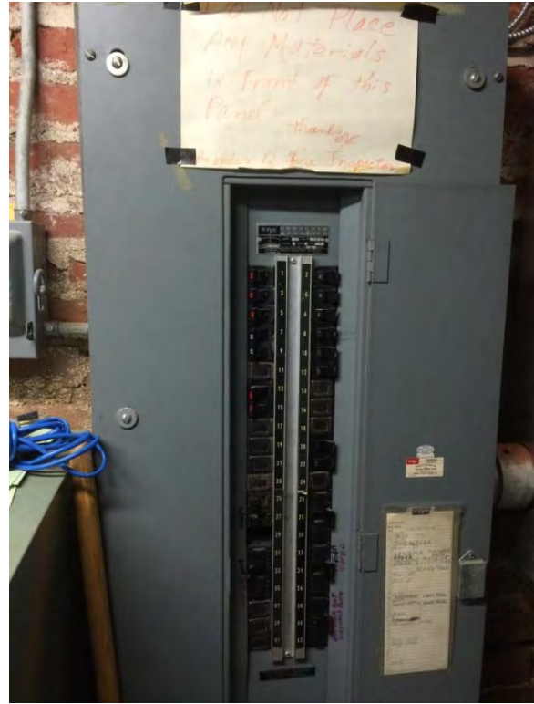
Figure 5.17: Library, main breaker panel.
