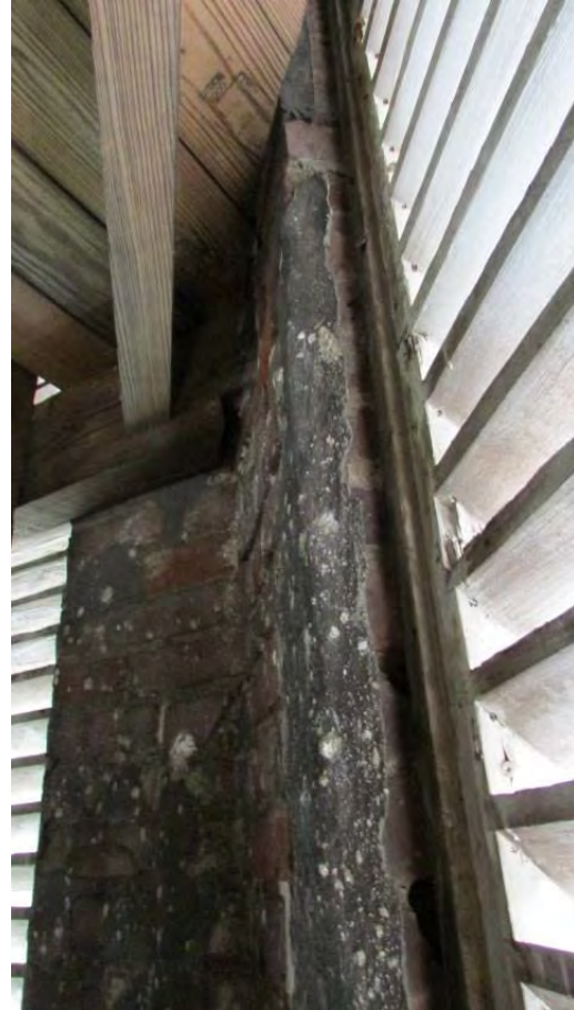
Figure 16: Weakened frame connections to jamb at louvers
