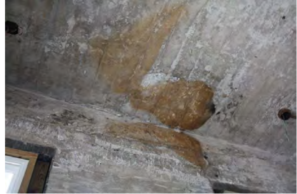
Figure 3.439, Old Jail, Second Floor, Room 201, view of moisture staining at the ceiling.
