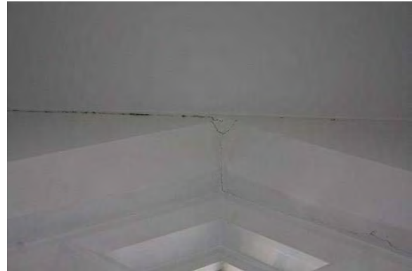
Figure 3.174, Historic Courthouse, Second Floor, Room 217, view of crack in plaster at head of window.
