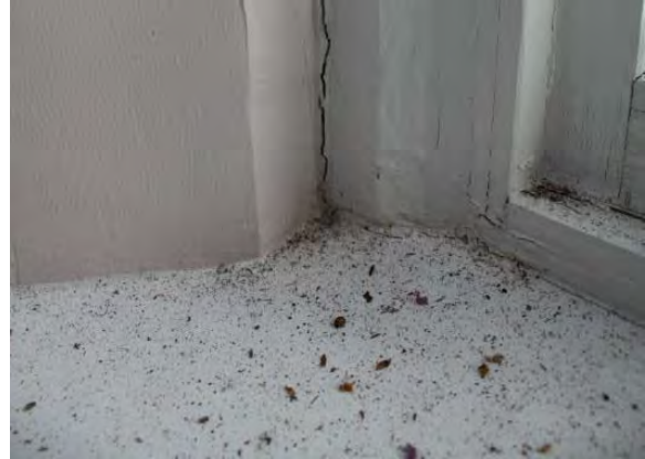
Figure 3.129, Historic Courthouse, Second Floor, Room 203, view of northernmost window at west wall; note the heavily-soiled sill and separation between the reveal and frame.
