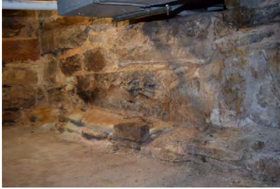
Figure 4.10: Large stone foundation walls under north wing with projecting footings at base
