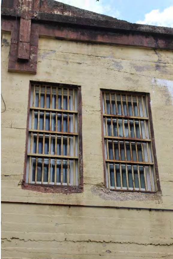
Figure 3.326, Old Jail, west elevation, view of typical second-story windows at the high-roofed south section. Note the concrete spalling where the sills are missing.
