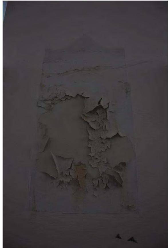
Figure 3.113, Historic Courthouse, First Floor, Room 132 (Stairway 2), view of paint failure due to moisture between the windows at the north wall.
