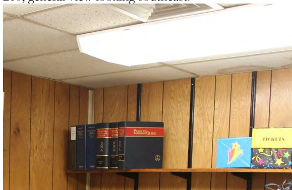
Figure 3.315, Old Wallace Library, Second Floor, Room 210, view of moisture staining at a ceiling tile.
