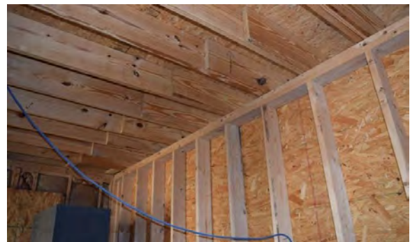
Figure 4.83: Northern Addition roof joists bearing on interior wood wall near building centerline
