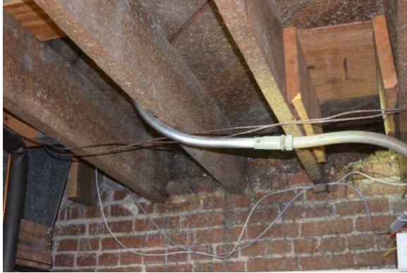
Figure 4.58: First floor framing at west end of mechanical room. Note evidence of mold.
