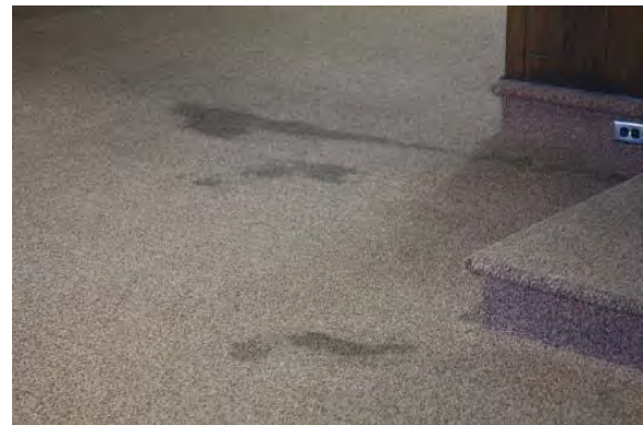
Figure 3.156, Historic Courthouse, Second Floor, Room 212, view of stains at the carpet adjacent to the judge's bench.
