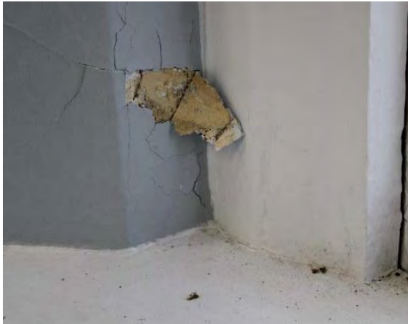
Figure 3.170, Historic Courthouse, Second Floor, Room 216, view of plaster damage due to efflorescence at the northernmost window of the west wall.
