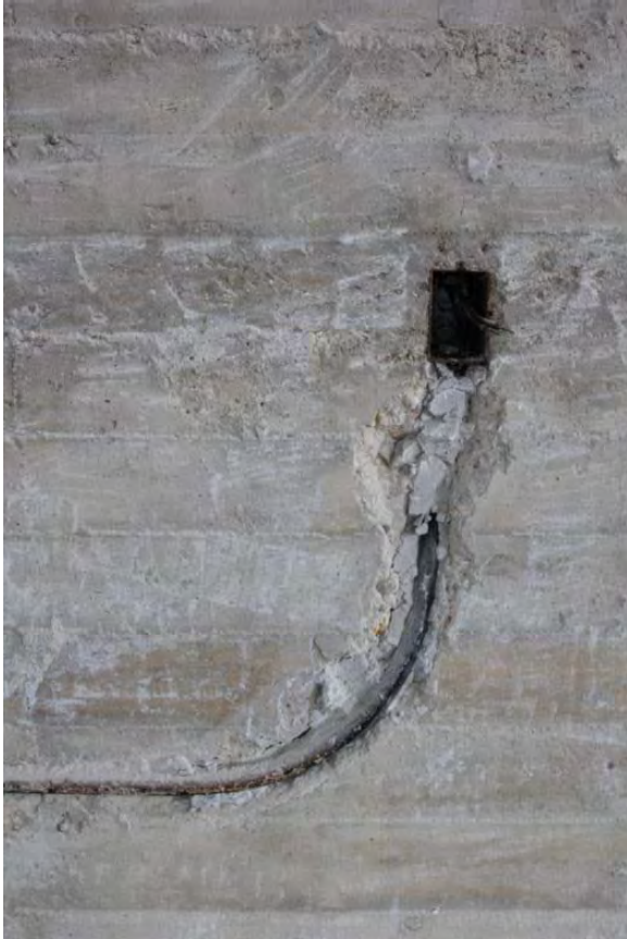
Figure 3.440, Old Jail, Second Floor, Room 201, view of remnants of a former electrical outlet and conduit at the north wall.
