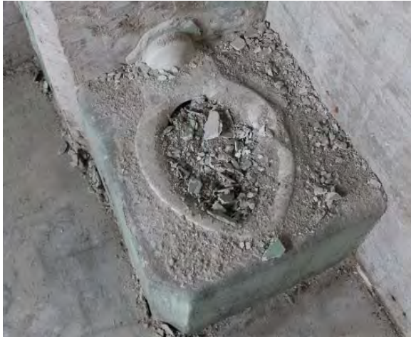
Figure 3.418, Old Jail, First Floor, Room 107, view of toilet filled with debris.
