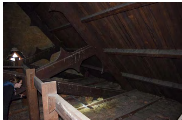
Figure 4.29: Scissor trusses supporting south wing roof with added 2 nd floor ceiling framing visible
