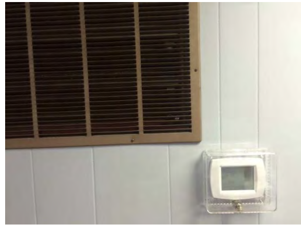
5.12: Library corridor return and thermostat.
