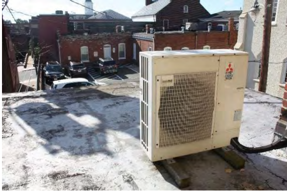
Figure 3.321, Old Jail, roof, view of sloped membrane roof at the one-story south wing.
