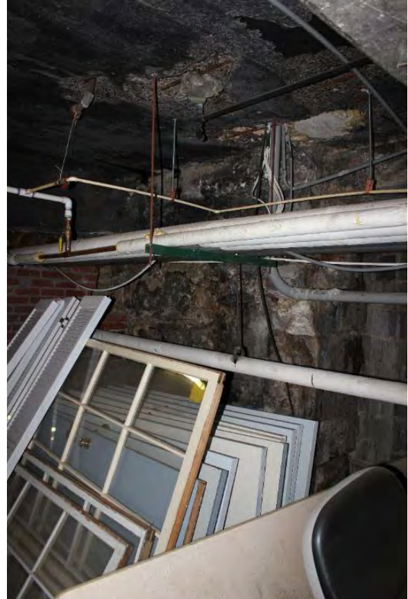
Figure 3.365, Old Jail, Basement, Room 003, general view looking southwest. Note the area of concrete block wall, which exhibits efflorescence and moisture staining.
