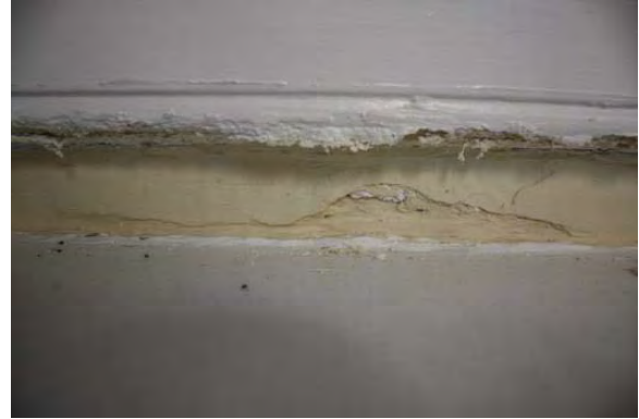
Figure 3.92, Historic Courthouse, First Floor, Room 123, view of plaster damage underneath the apron of the west window of the north wall.
