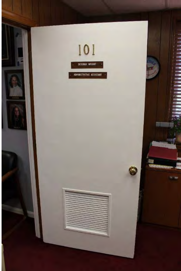
Figure 3.279, Old Wallace Library, First Floor, Room 105, view of typical first-story, hollow-core wood door.
