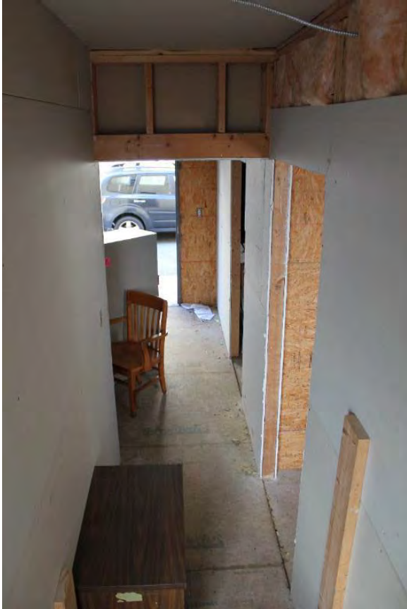
Figure 3.426, Old Jail, First Floor, Room 109, general view looking west from stair hall. Note the exposed insulation along the top of the north wall.
