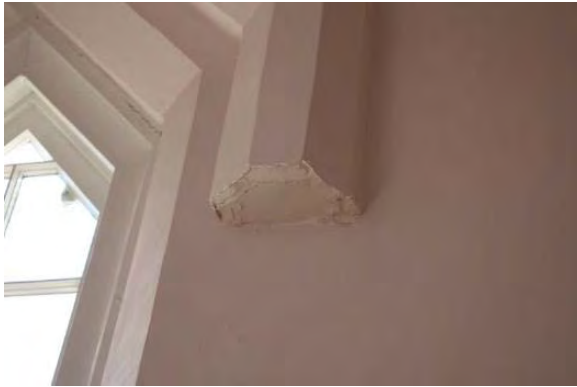
Figure 3.144, Historic Courthouse, Second Floor, Room 211, view of missing pendant at window hood mold.
