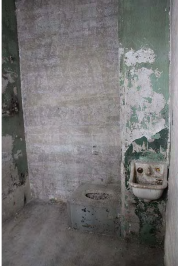
Figure 3.410, Old Jail, First Floor, Room 106, view looking west. Note the heavy paint loss at the walls.
