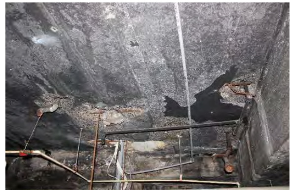
Figure 3.366, Old Jail, Basement, Room 003, view of the poured-in-place concrete ceiling. Note the areas of loss, patching, and exposed, rusted rebar and rusted pipes.
