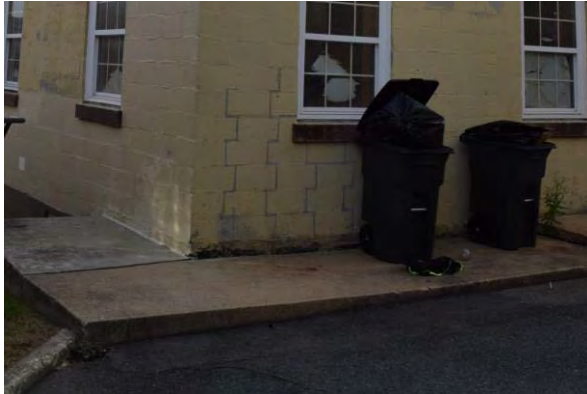
Figure 4.63: Settlement of the concrete sidewalk at northwest corner. Note also the previous repointing efforts in CMU walls.
