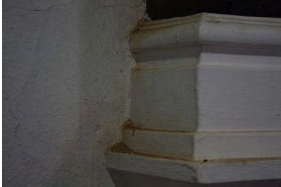
Figure 3.153, Historic Courthouse, Second Floor, Room 212, view of dust from masonry wall adjacent to a pendant post in the northwest corner of the room; this is evidence of efflorescence.
