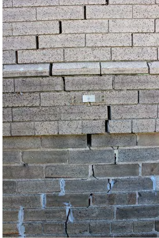
Figure 1.11, Wallace Library. Pervasive shifting and cracking of brick in the north elevation. Photograph 2015.
