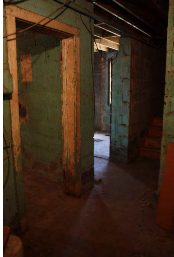
Figure 3.372, Old Jail, Basement, Room 004, general view looking northeast. Note the heavy paint loss at the door frame leading to Room 005.
