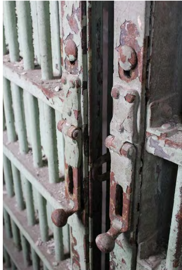
Figure 3.419, Old Jail, First Floor, Room 107, detail view of jail cell doors. Note the heavy paint loss and rust.
