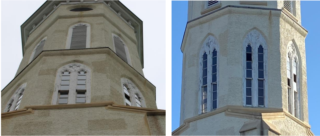
Figure 2: At Left, August 2020 Image Showing Missing Glass in Tower Windows; at Right, April 2023 Image Depicting Further Deterioration with Loss of Additional Panes and Loosened/Failing Components of Original Wood Window Frames.
